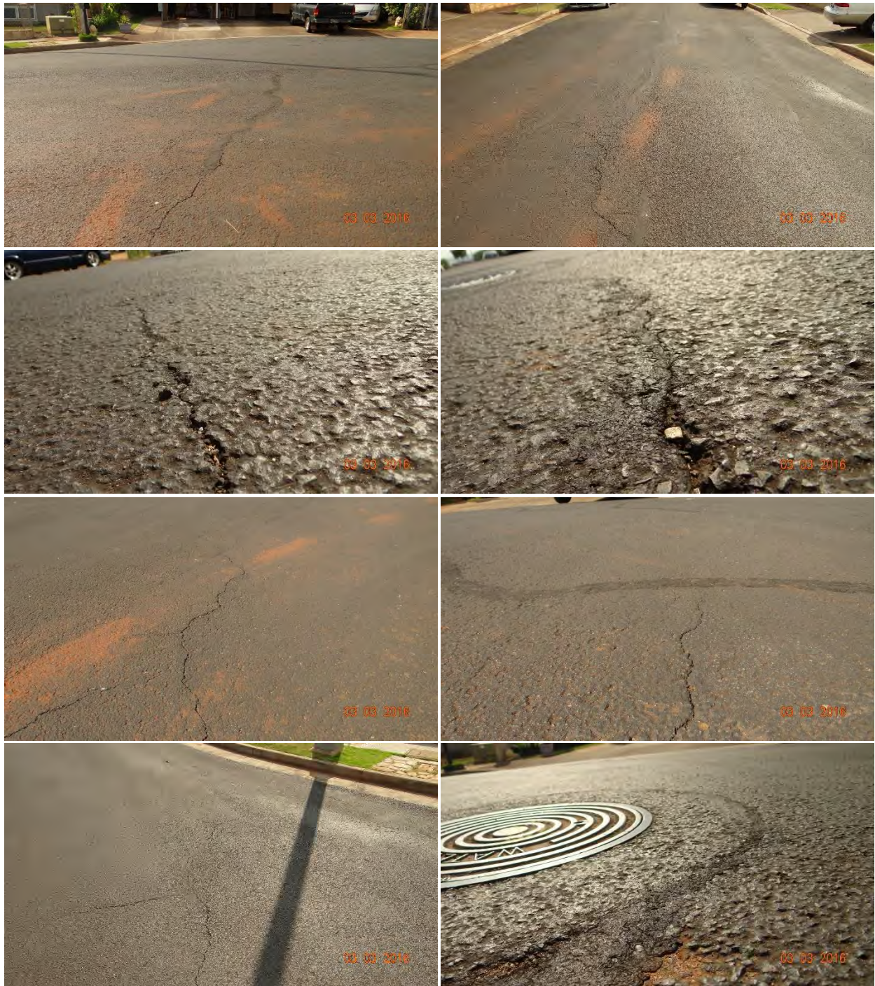
Figure C-120 Condition of the section on Hoolana Place, treated with OptiPave Plus™ Ready to Use by SealMasters®/Hawaii, on 3/3/2016.
