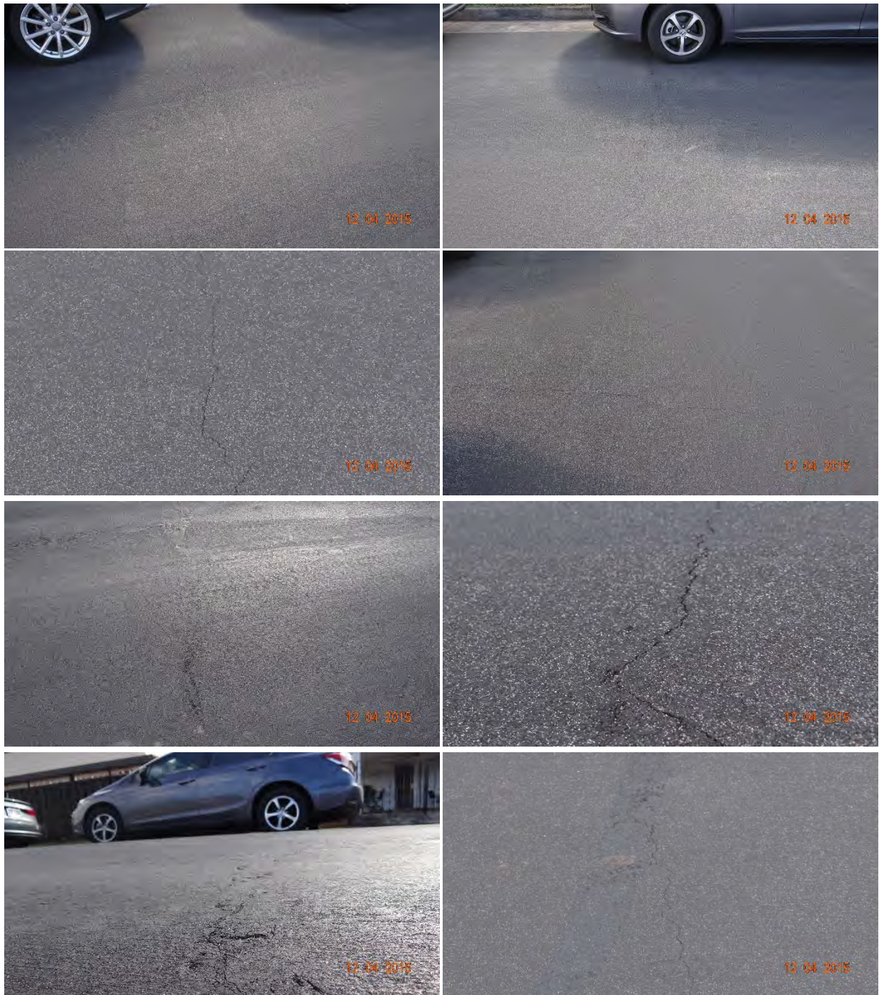
Figure C-62 Condition of Kaweloka Street section 2, treated with Liquid Road, on 12/4/2015.
