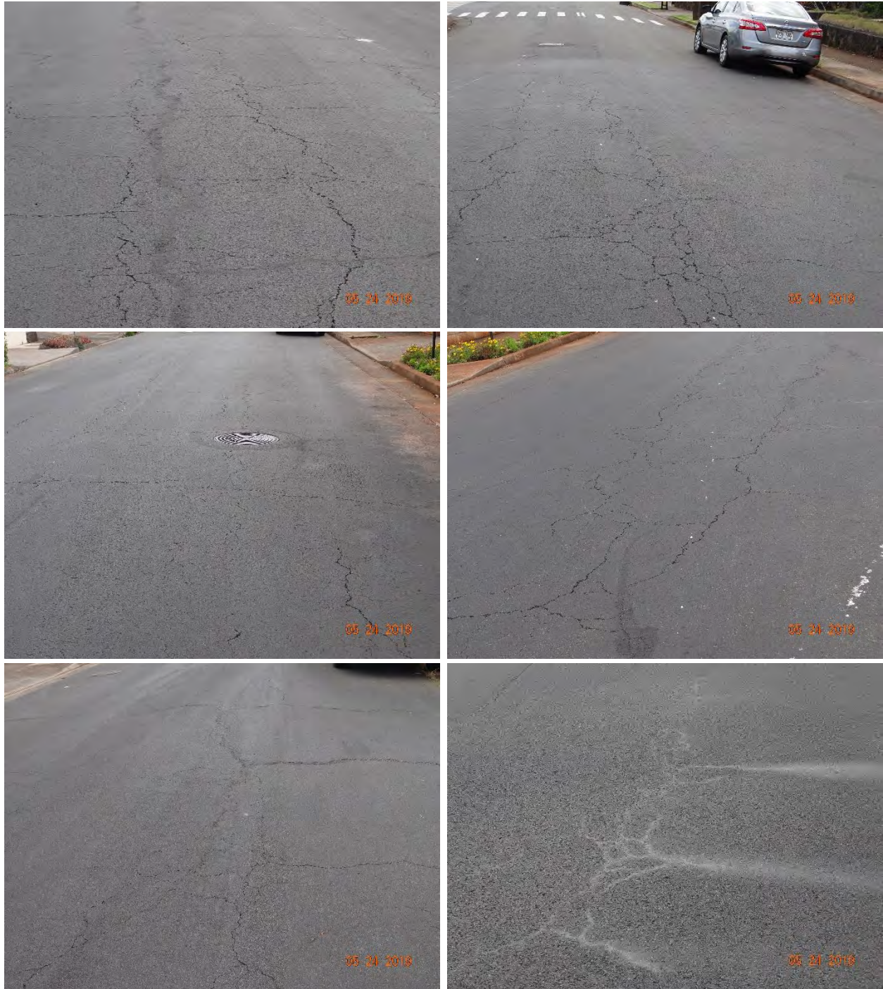
Figure 4-33 Fatigue cracking progression in the sections with bus traffic.
