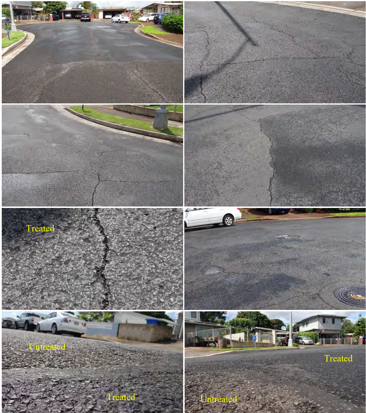
Figure C-123 Condition of the section on Hoolana Place, treated with OptiPave Plus™ Ready to Use by SealMasters®/Hawaii, on 2/7/2018.
