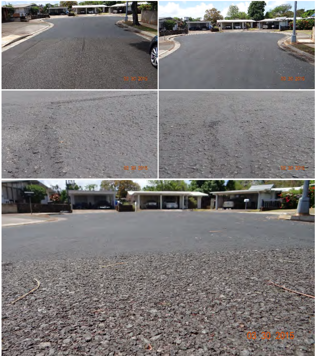
Figure C-134 Condition of the section on Hooheho Place, before treatment with CarbonSeal-HF by Carbonyte Systems Inc., on 3/30/2015.
