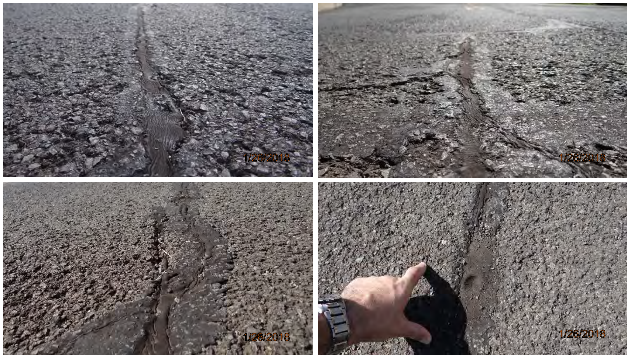
Figure C-20 Condition of crack sealing observed on Hookano Street on 01/26/2018 (sealed with Roadsaver 211).
