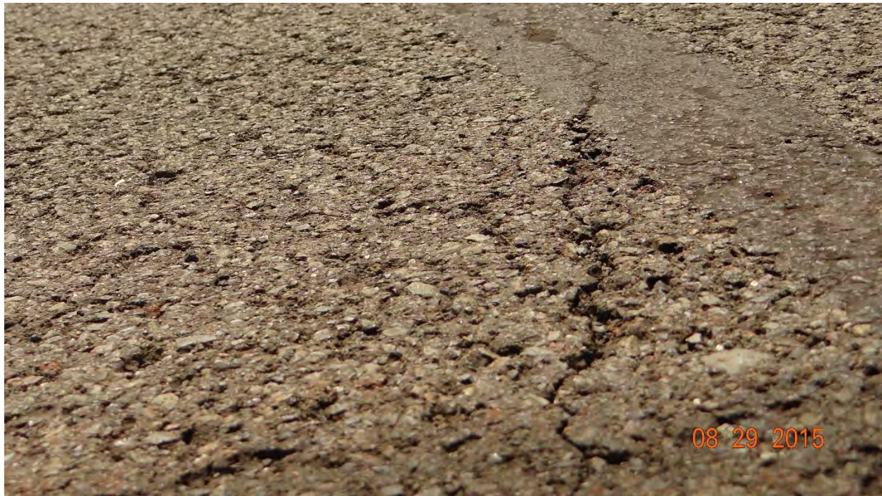
Figure C-12 Condition of crack sealing observed on Hookano Street on 08/29/2015 (sealed with Roadsaver 211).
