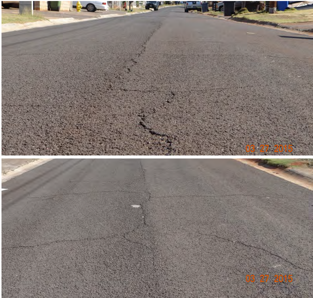
Figure C-2 Cracking patterns observed on the Control Section on Hoolauna Street on 03/03/2015.
