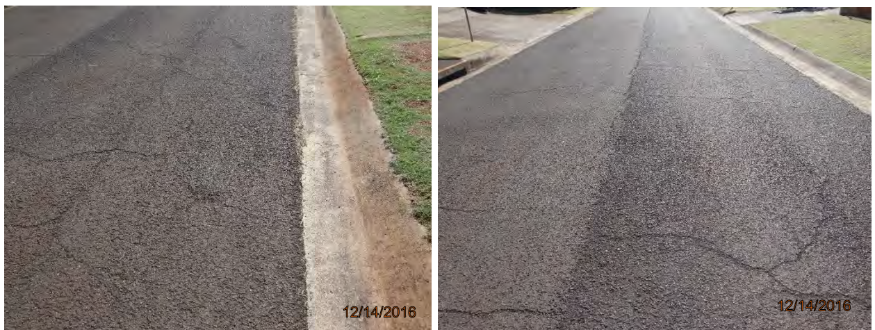
Figure C-4 Cracking patterns observed on the Control Section on Hoolauna Street on 12/14/2016.
