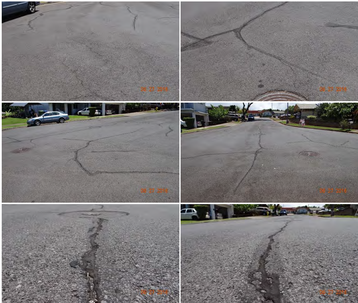
Figure C-41 Condition of the Paaaina Place section on 06/27/2016.
