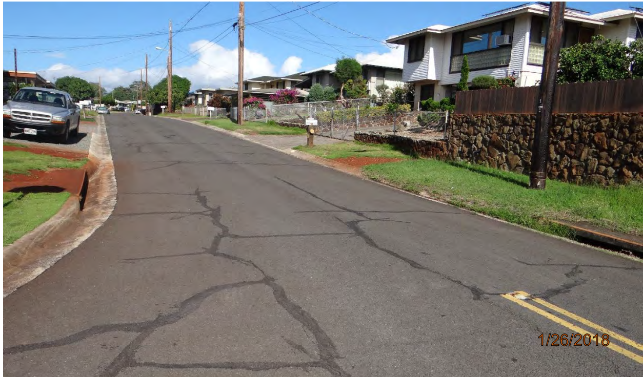
Figure C-21 Condition of crack sealing observed on Hookano Street on 01/26/2018 (sealed with Roadsaver 211).
