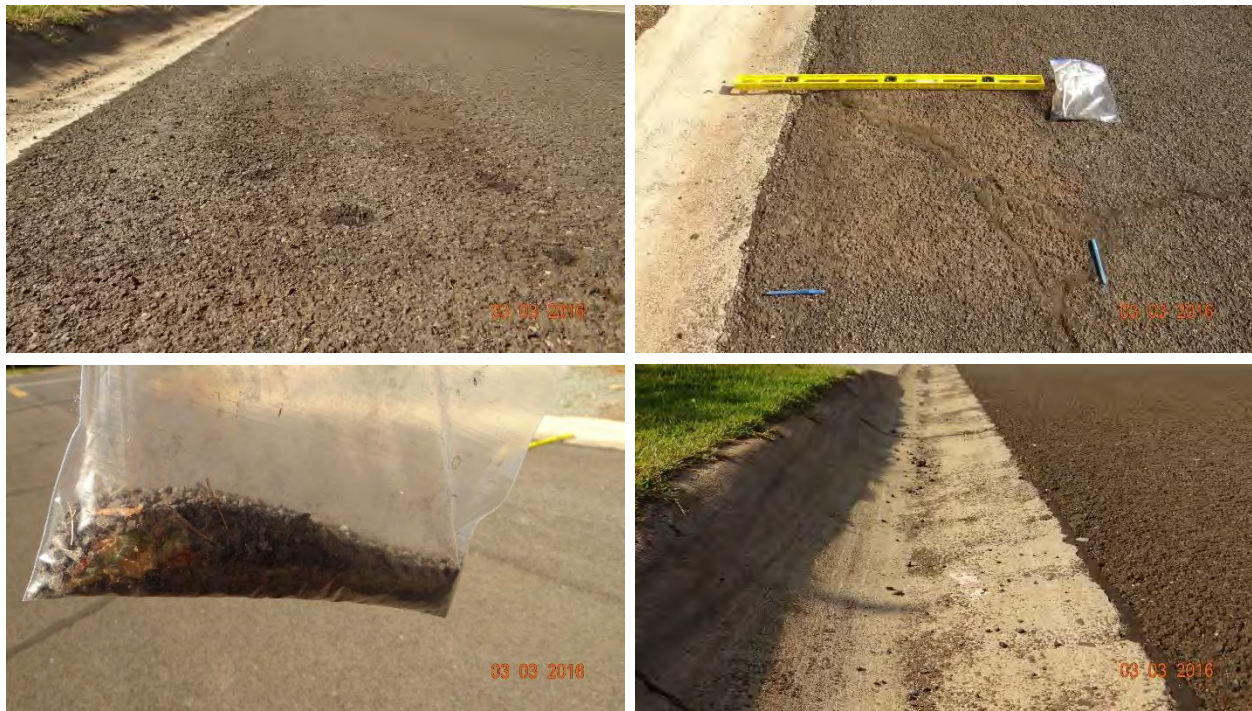
Figure C-14 Raveling observed on Hookano Street on 03/03/2016 (sealed with Roadsaver 211).
