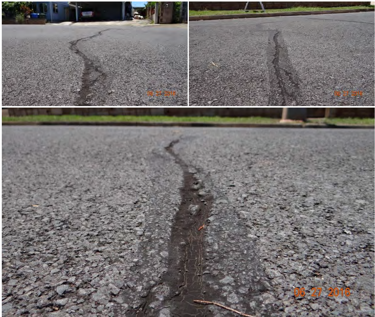
Figure C-42 Condition of the Paaaina Place section on 06/27/2016.
