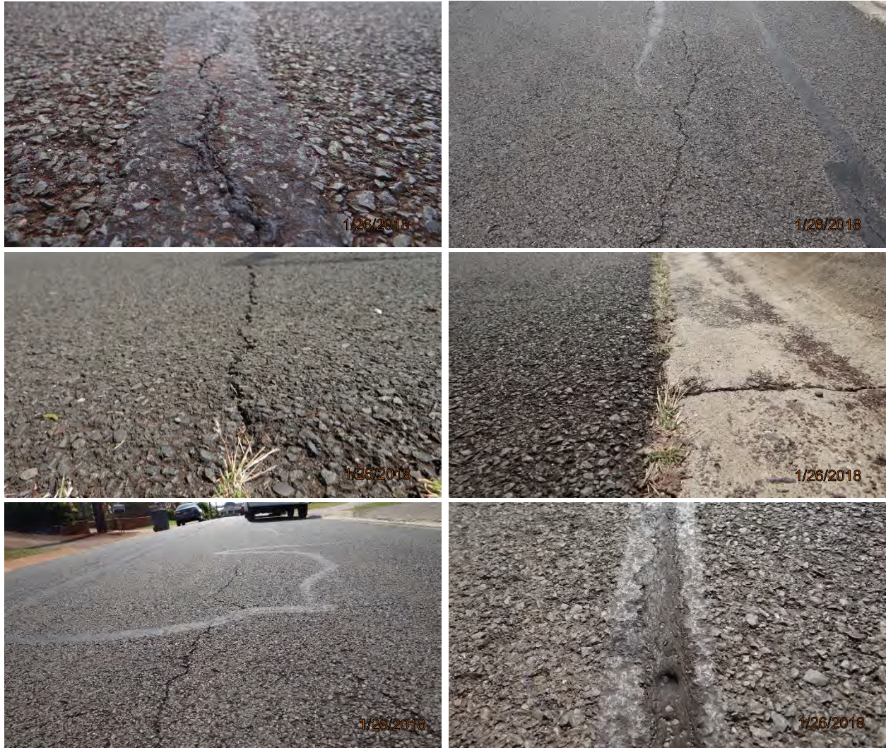
Figure C-9 Condition of crack sealing observed on Hoowali Street on 01/26/2018 (sealed with CrackMaster™ PL-HT).
