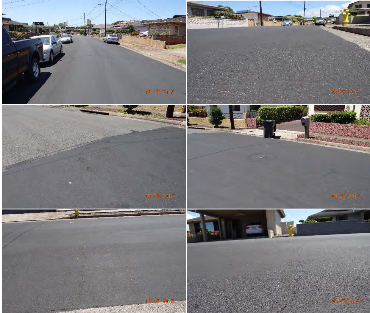
Figure C-60 Condition of Kaweloka Street section 2, treated with Liquid Road, on 3/27/2015.
