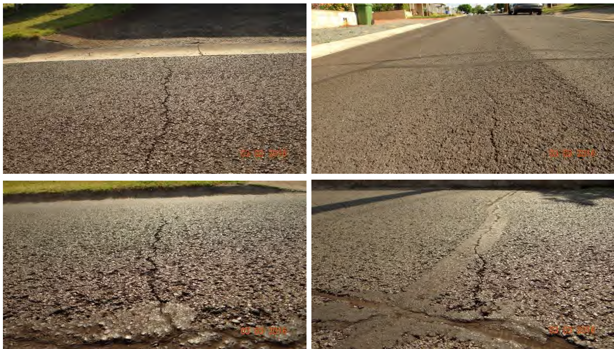
Figure C-15 Condition of crack sealing observed on Hookano Street on 03/03/2016 (sealed with Roadsaver 211).
