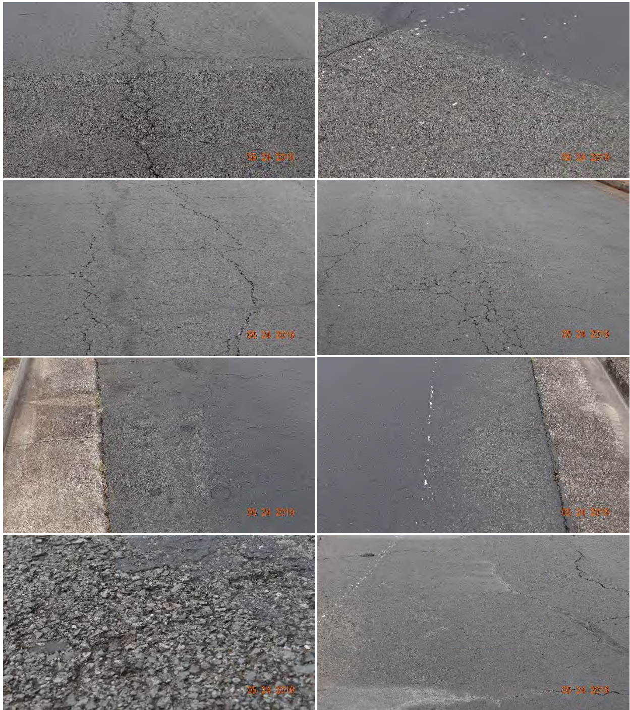
Figure C-82 Cracking on Kaweloka Street section 4, treated with OptiPave Plus™ RTU, on 5/24/2019.
