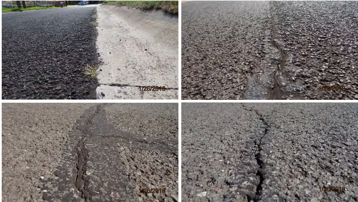
Figure C-18 Condition of crack sealing observed on Hookano Street on 01/26/2018 (sealed with Roadsaver 211).
