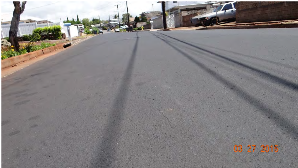
Figure C-76 Condition of Kaweloka Street section 4, treated with OptiPave Plus™ RTU, on 3/27/2015.
