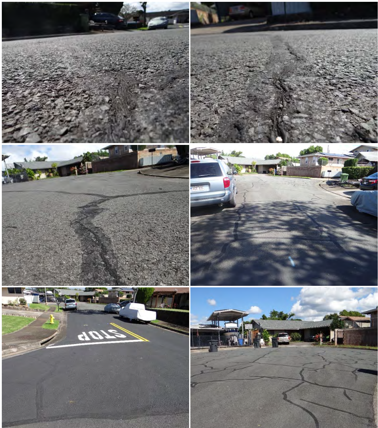
Figure C-31 Condition of the Kaweloka Place section on 12/14/2016.
