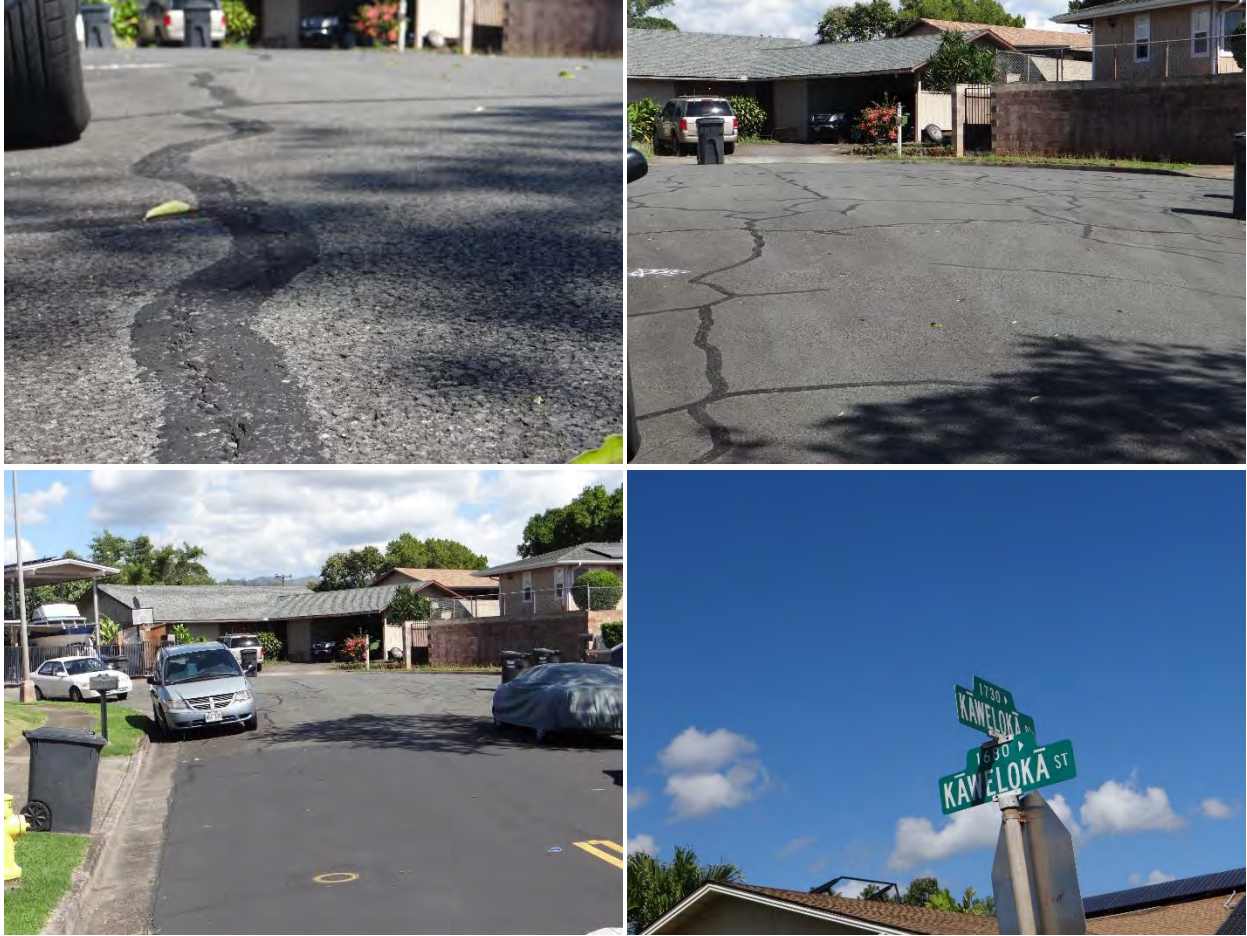
Figure C-34 Condition of the Kaweloka Place section on 01/26/2018.
