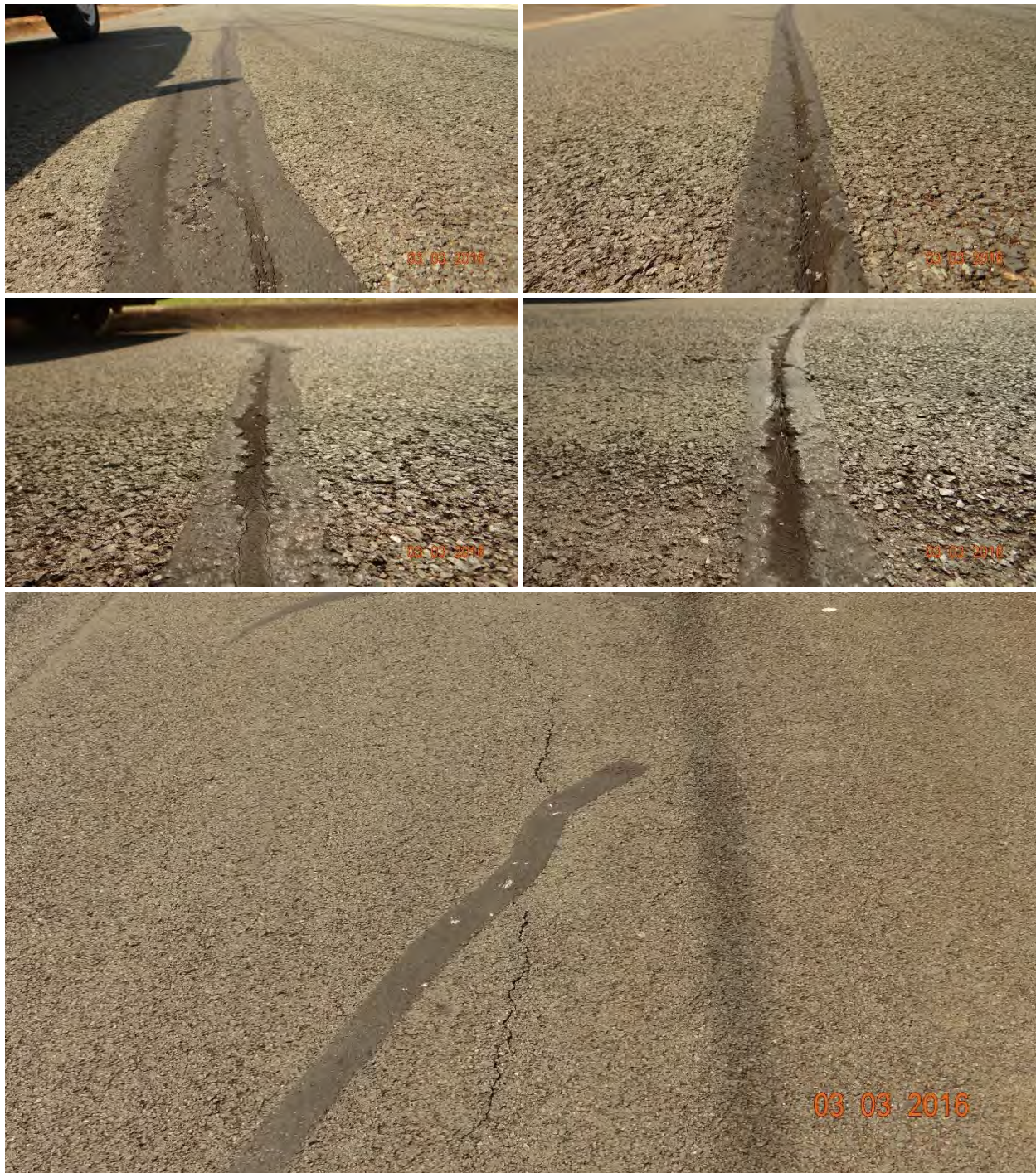
Figure C-6 Condition of crack sealing observed on Hoowali Street on 03/03/2016 (sealed with CrackMaster™ PL-HT).
