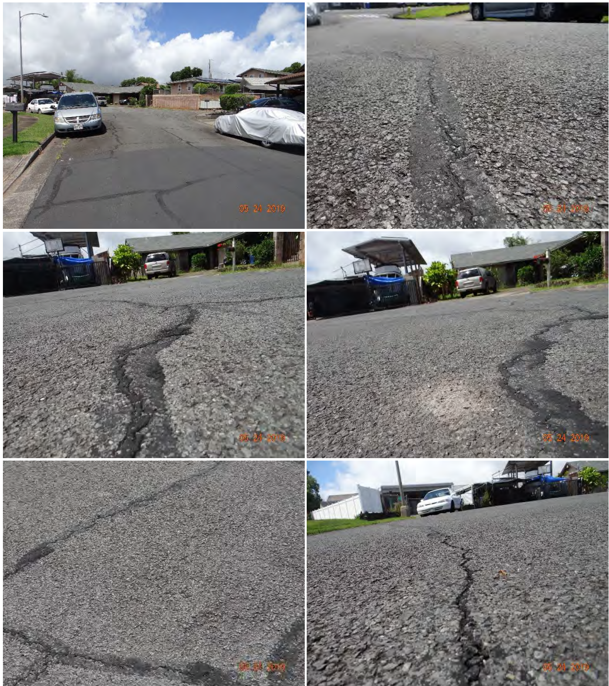
Figure C-35 Condition of the Kaweloka Place section on 5/24/2019.
