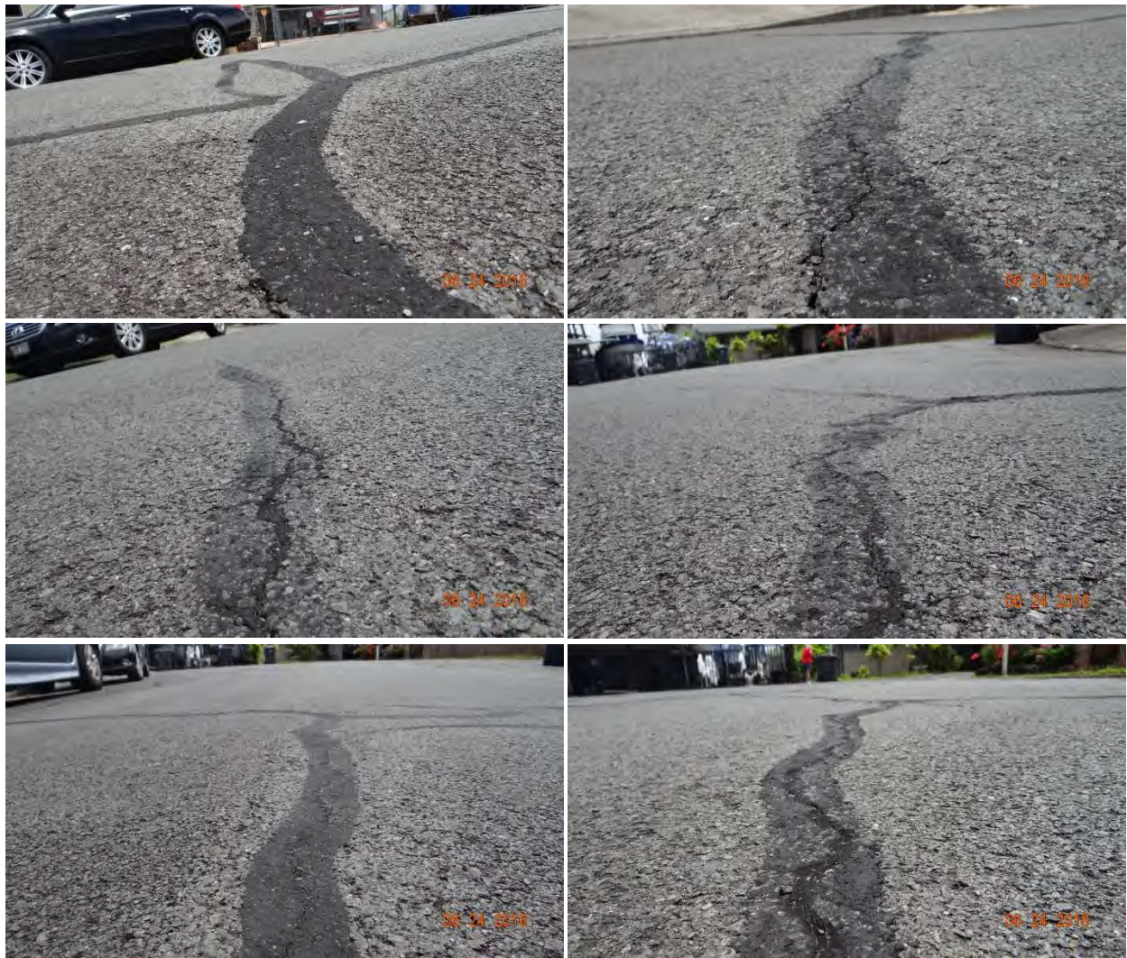
Figure C-29 Condition of the Kaweloka Place section on 06/24/2016.
