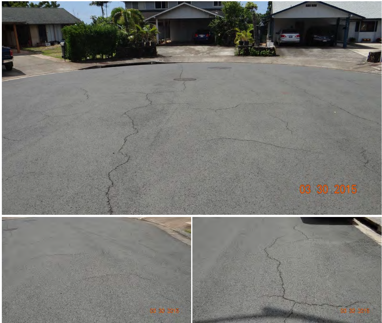
Figure C-23 Condition of the Palamoi Street section on 03/20/2015 (three months into the study period) used as control for crack sealing.
