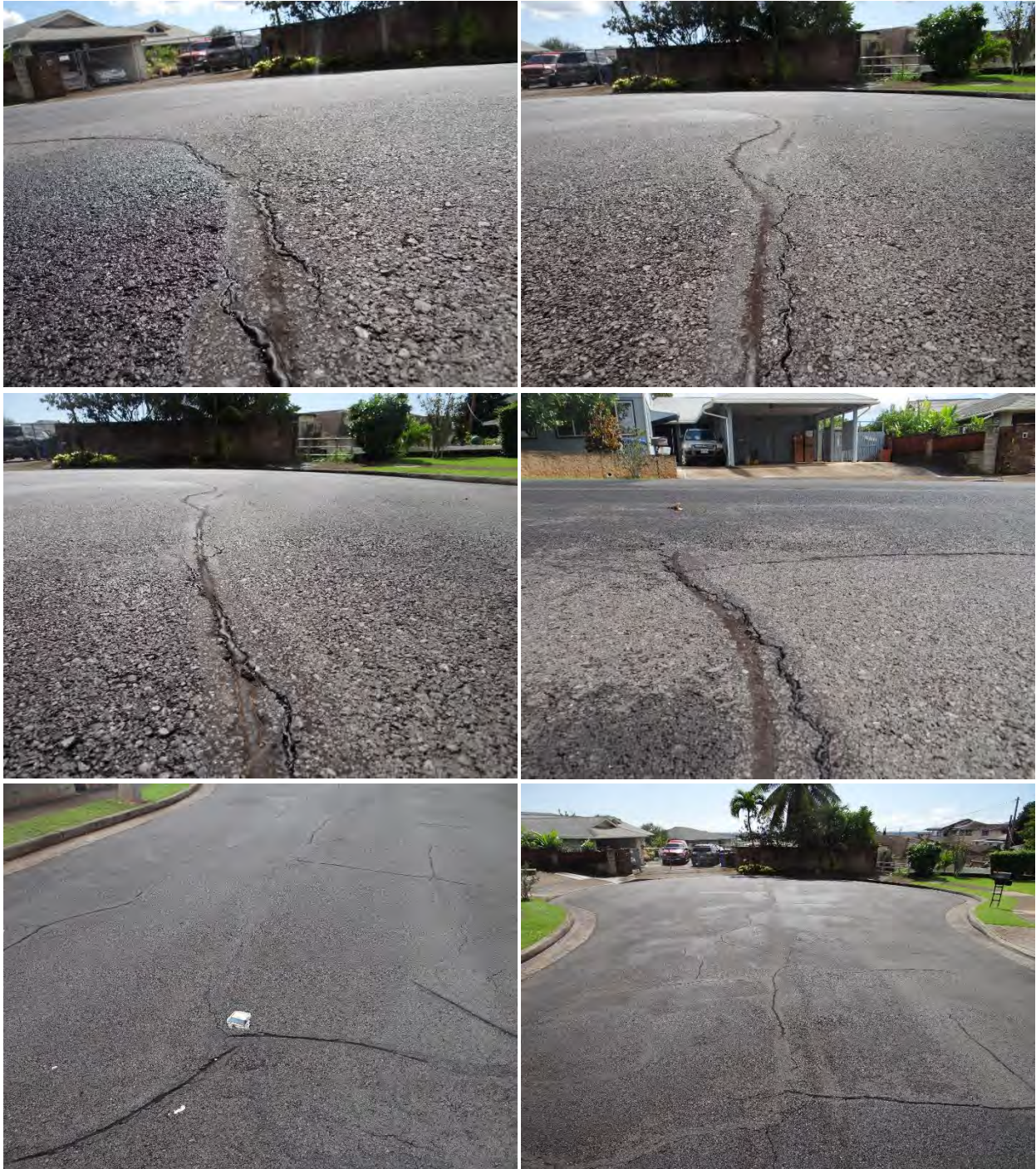
Figure C-45 Condition of the Paaaina Place section on 02/07/2018.
