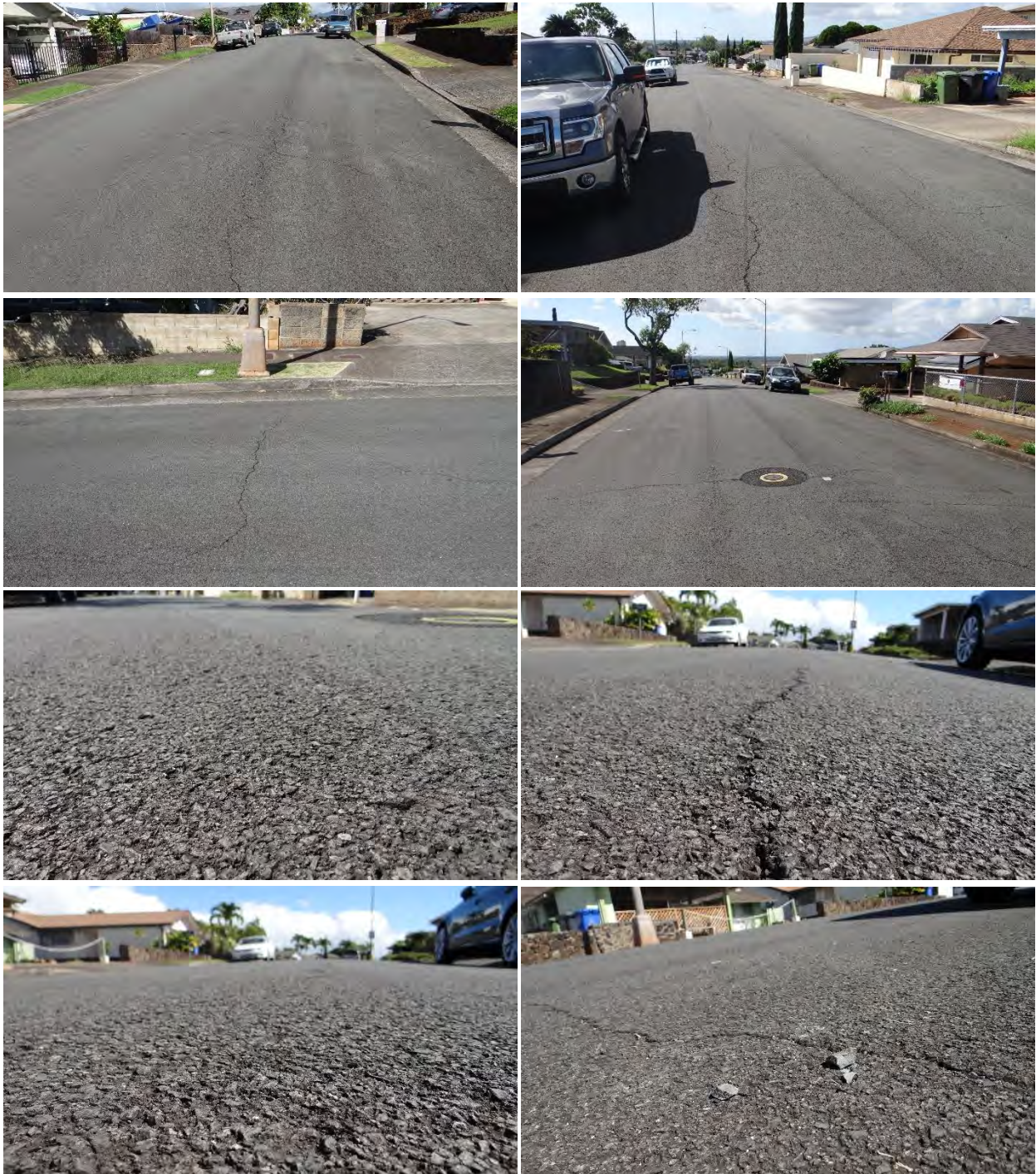
Figure C-85 Condition of control sections 6, 7, 8 for straight sections without bus traffic on Kaweloka Street, on 12/13/2016.
