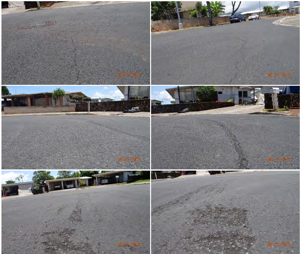
Figure C-135 Condition of the section on Hooheno Place, before treatment with CarbonSeal-HF by Carbonyte Systems Inc., on 6/27/2016.
