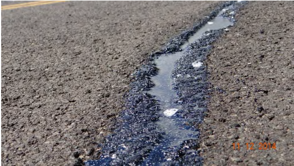
Figure 3-16 Sealed cracks were left slightly recessed.
