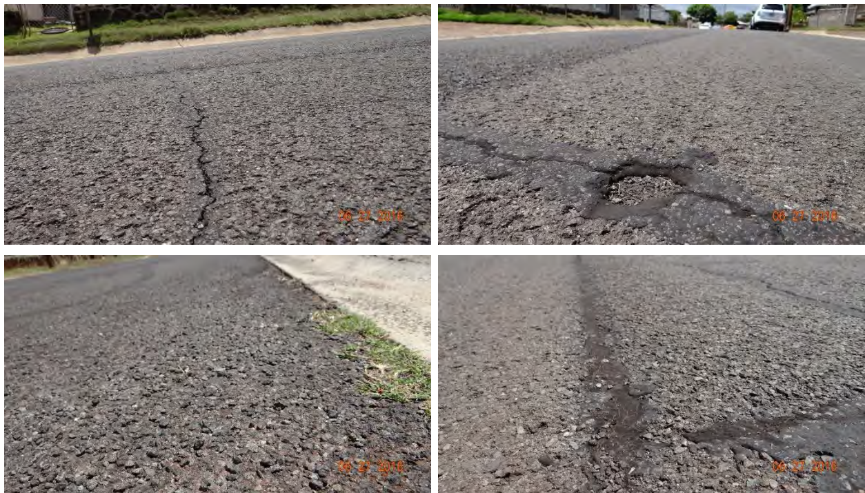
Figure C-17 Condition of crack sealing observed on Hookano Street on 06/27/2016 (sealed with Roadsaver 211).
