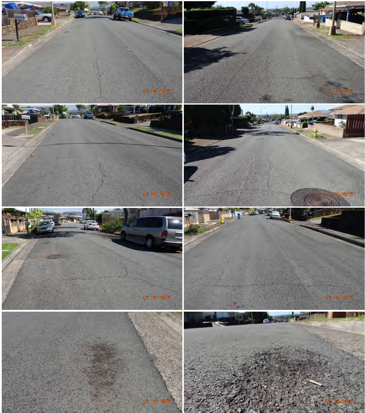
Figure C-83 Condition of control sections 6, 7, 8 for straight sections without bus traffic on Kaweloka Street, on 1/26/2015.
