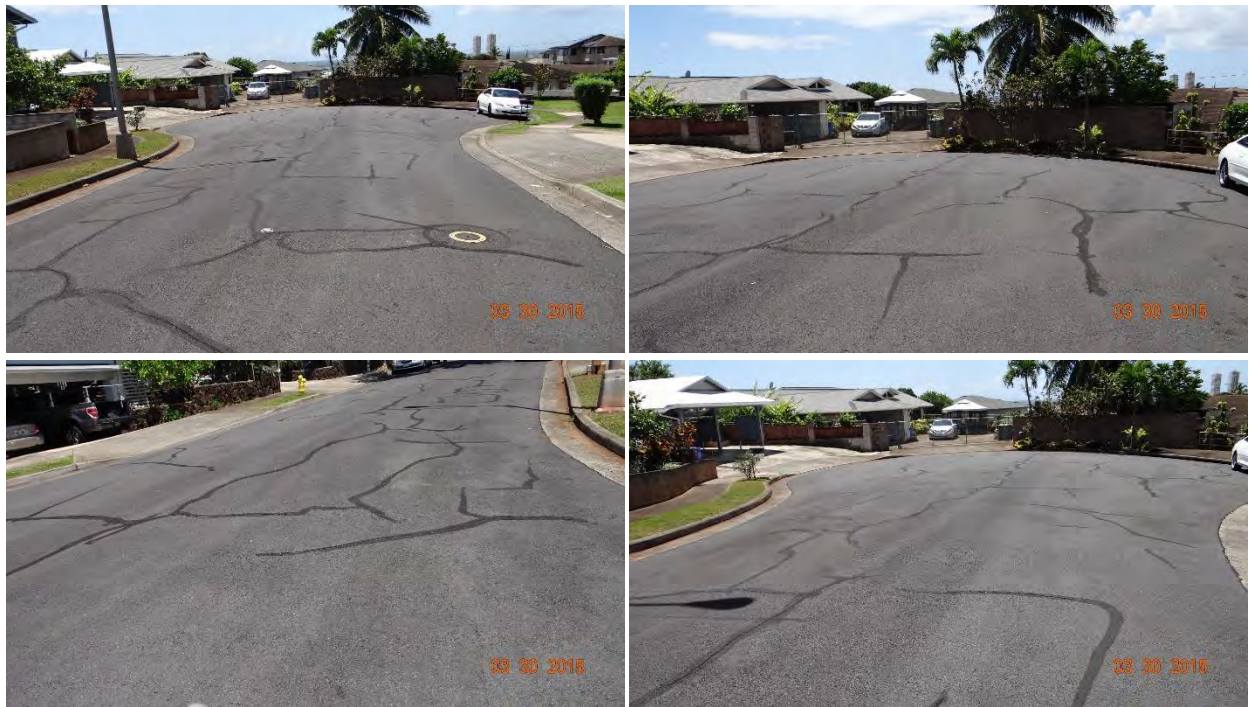
Figure C-36 Condition of the Paaaina Place section on 03/30/2015.
