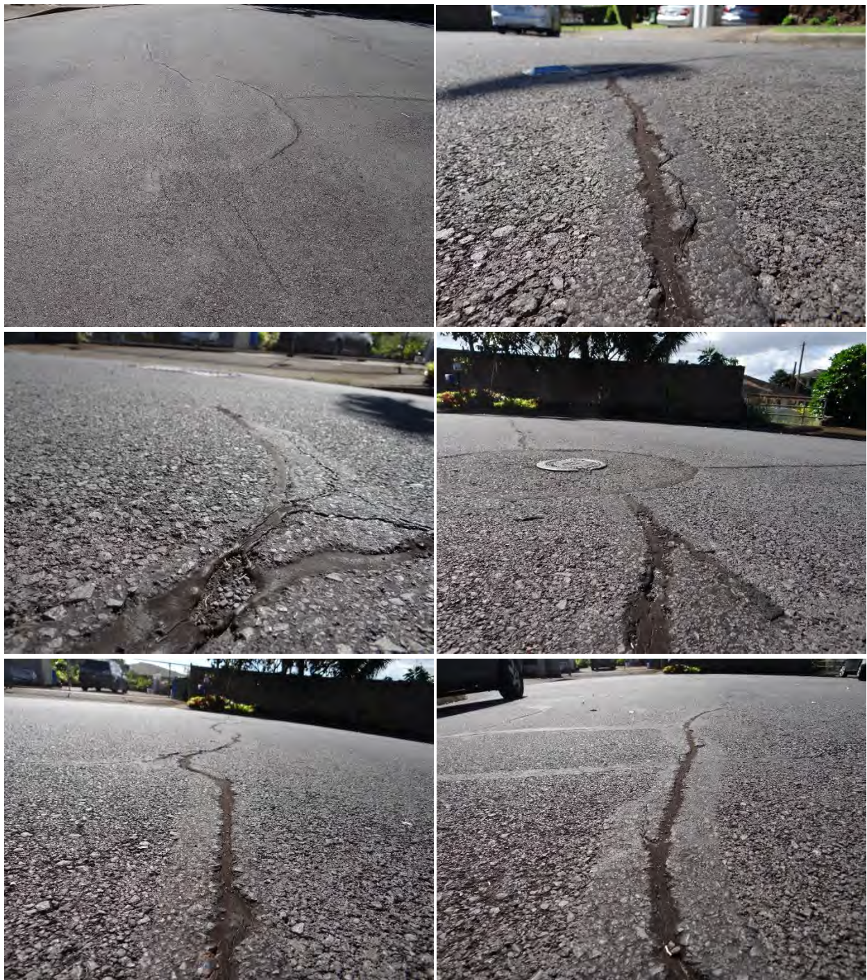
Figure C-43 Condition of the Paaaina Place section on 12/14/2016.
