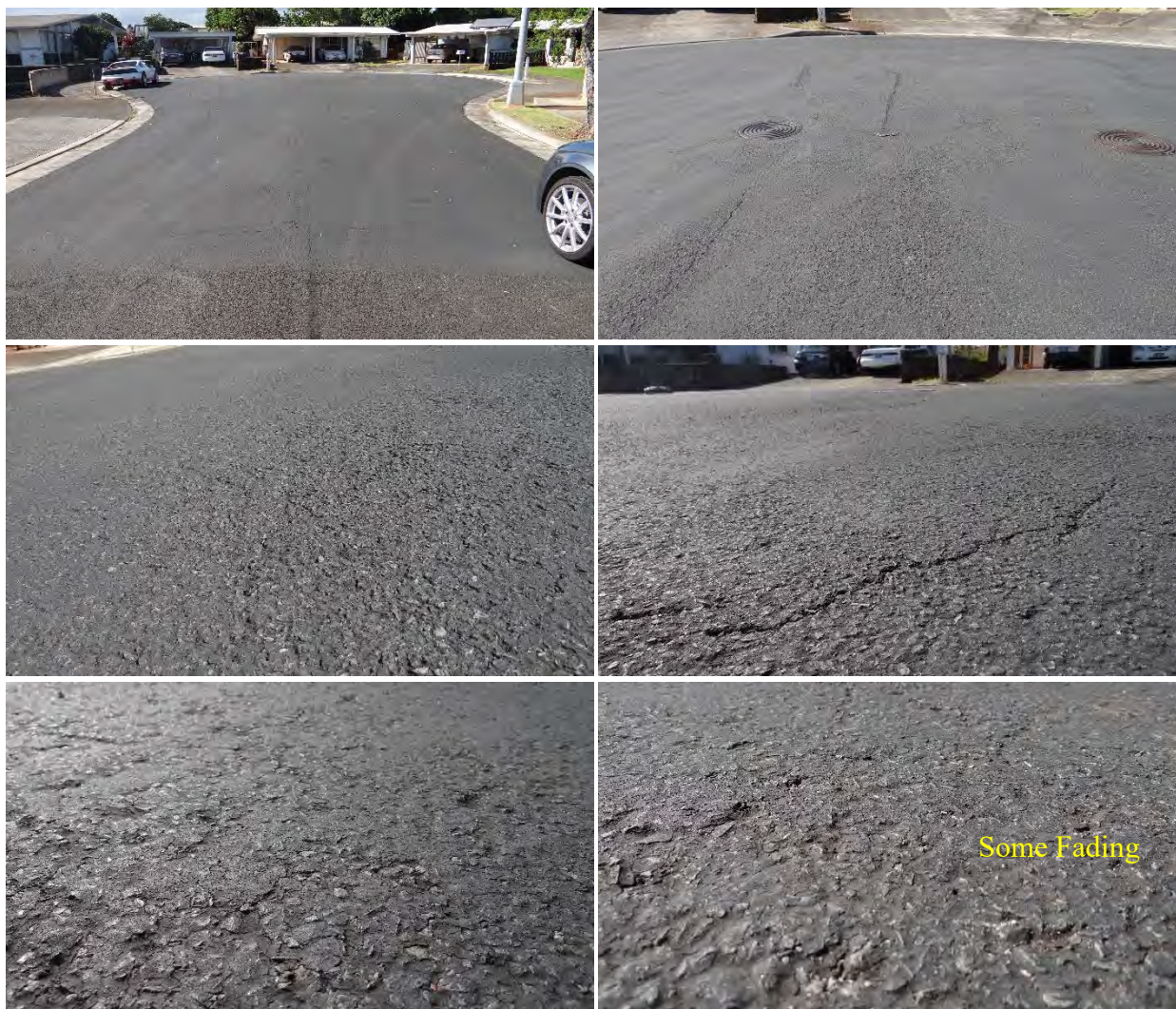
Figure C-136 Condition of the section on Hooheno Place, before treatment with CarbonSeal-HF by Carbonyte Systems Inc., on 12/14/2016.
