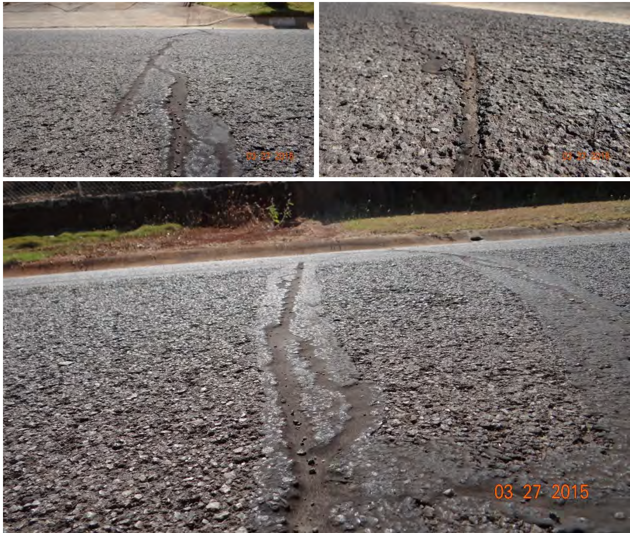
Figure C-11 Condition of crack sealing observed on Hookano Street on 03/27/2015 (sealed with Roadsaver 211).
