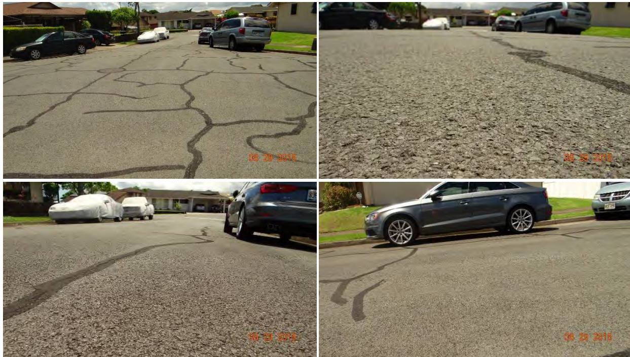
Figure C-25 Condition of the Kaweloka Place section on 08/29/2015.
