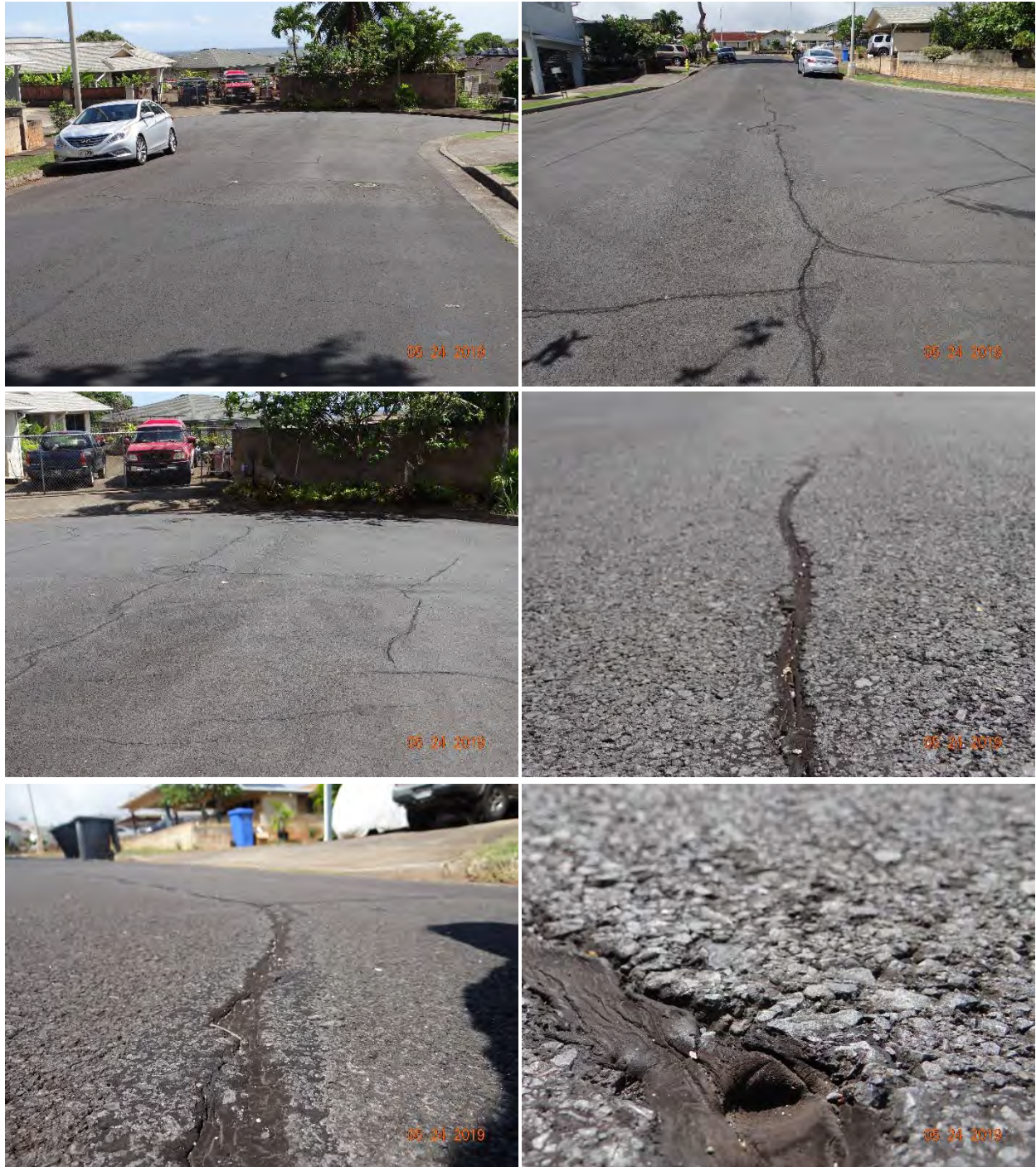
Figure C-49 Condition of the Paaaina Place section on 5/24/2019.
