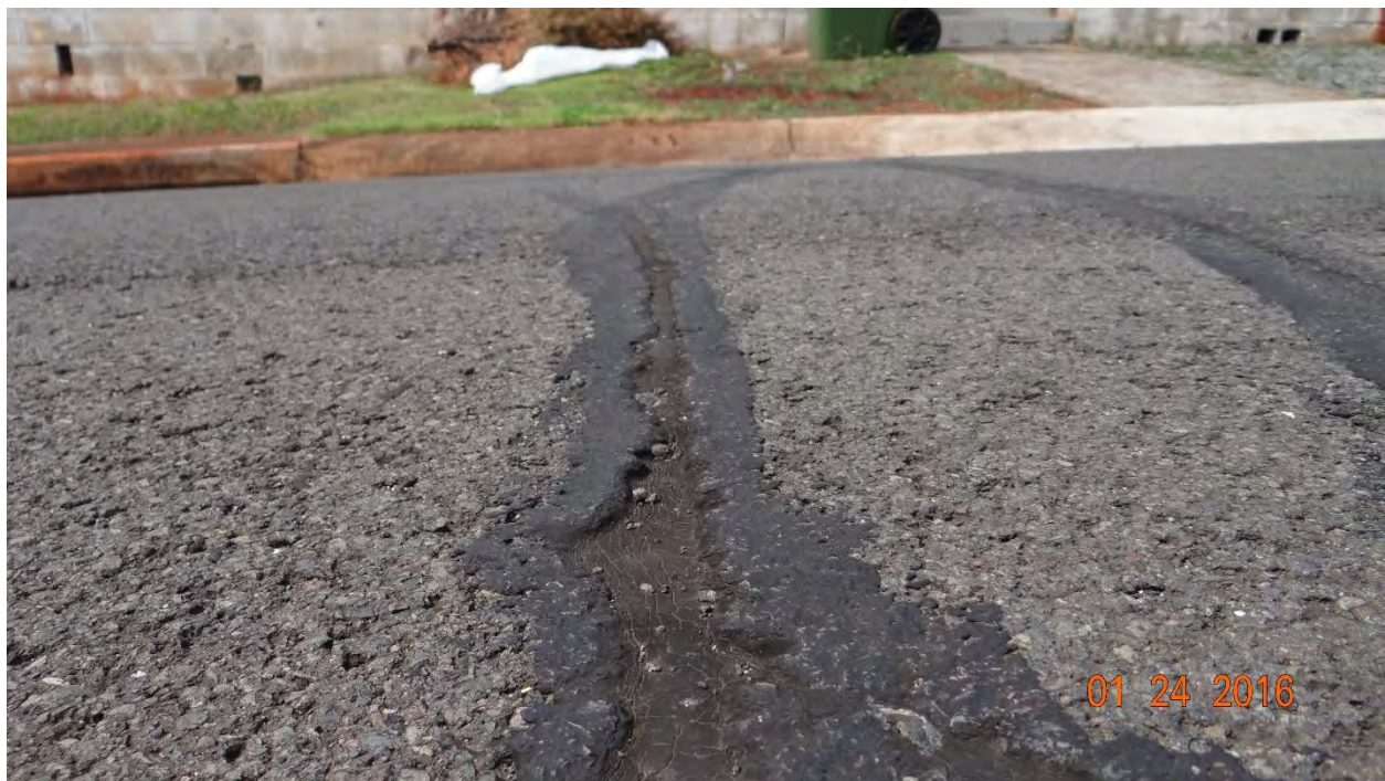
Figure C-13 Condition of crack sealing observed on Hookano Street on 01/24/2016 (sealed with Roadsaver 211).
