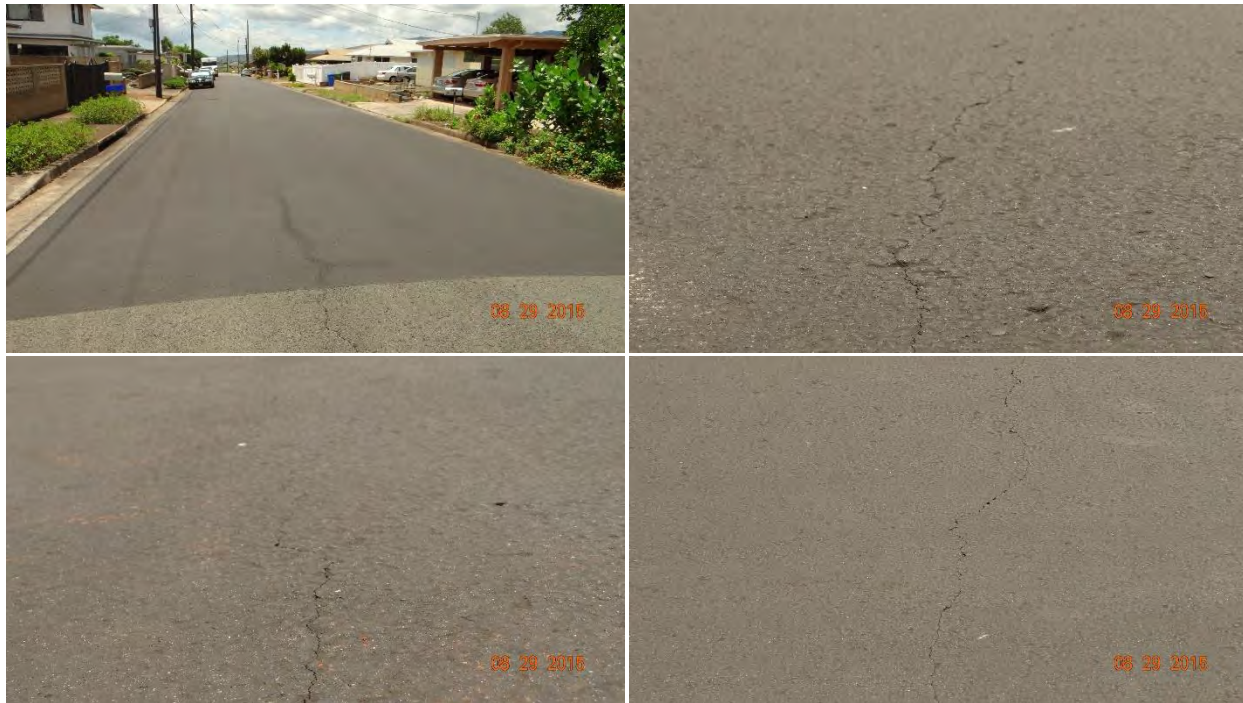
Figure C-77 Condition of Kaweloka Street section 4, treated with OptiPave Plus™ RTU, on 8/29/2015.
