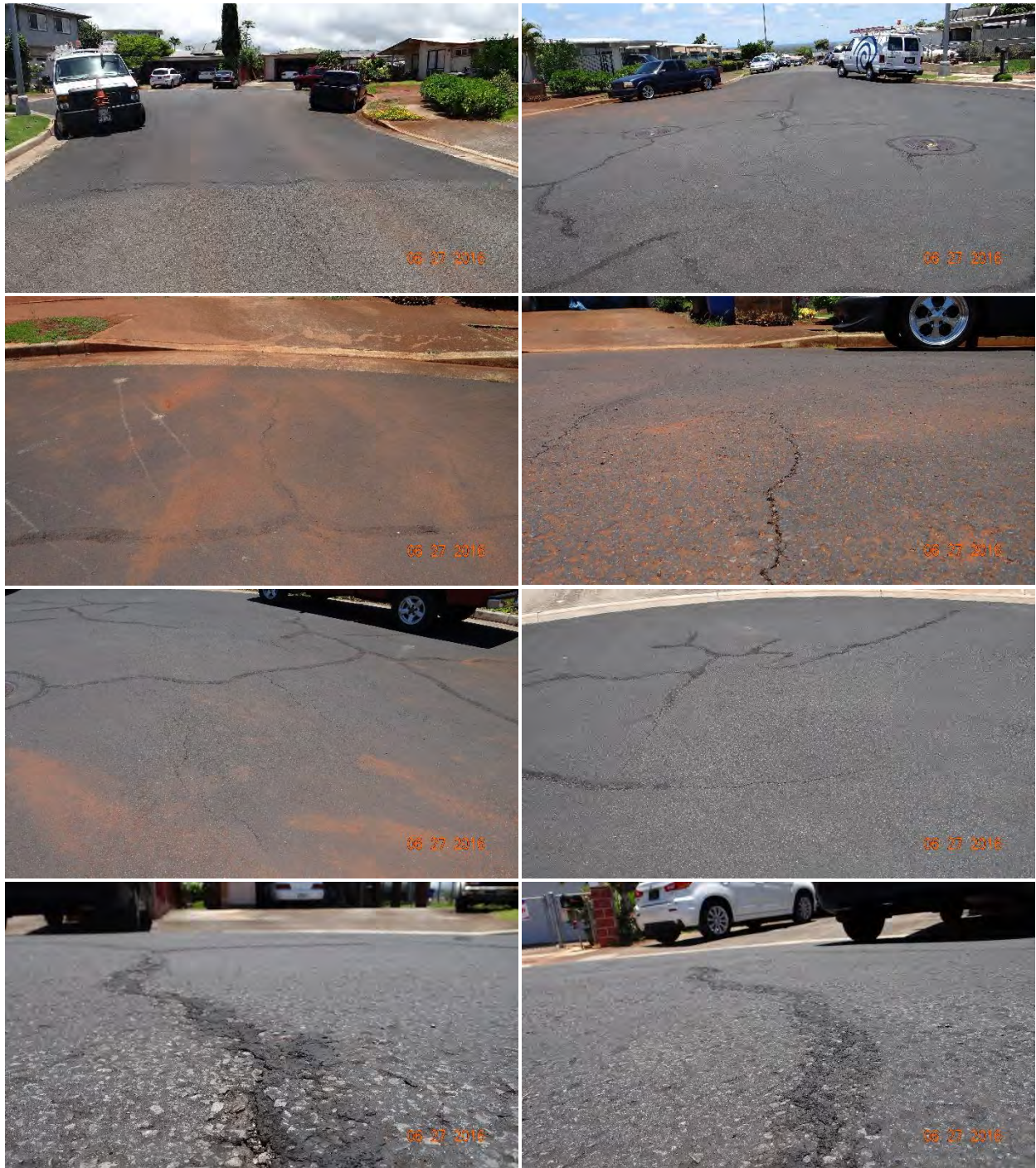
Figure C-121 Condition of the section on Hoolana Place, treated with OptiPave Plus™ Ready to Use by SealMasters®/Hawaii, on 6/27/2016.
