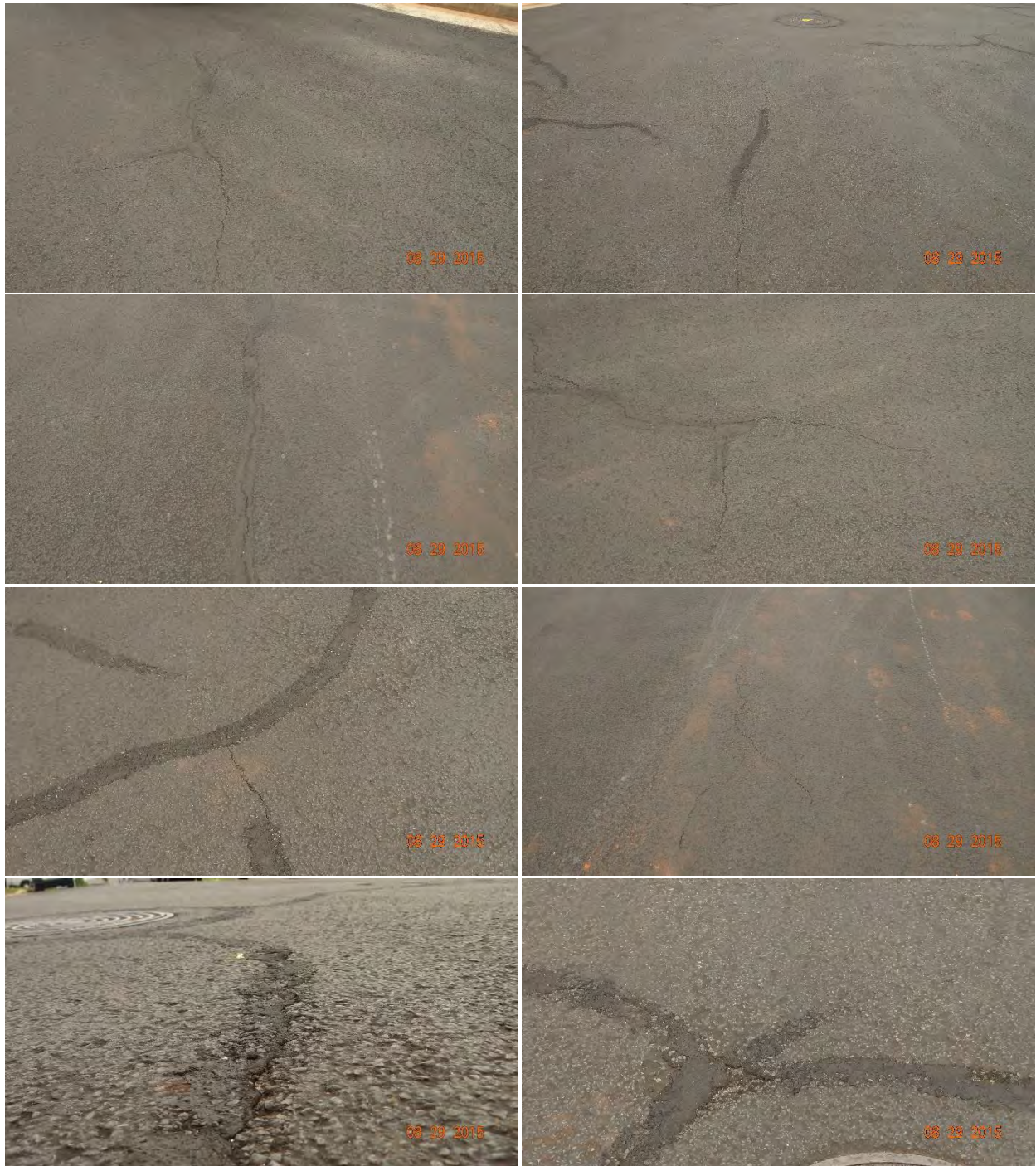
Figure C-119 Condition of the section on Hoolana Place, treated with OptiPave Plus™ Ready to Use by SealMasters®/Hawaii, on 8/29/2015.
