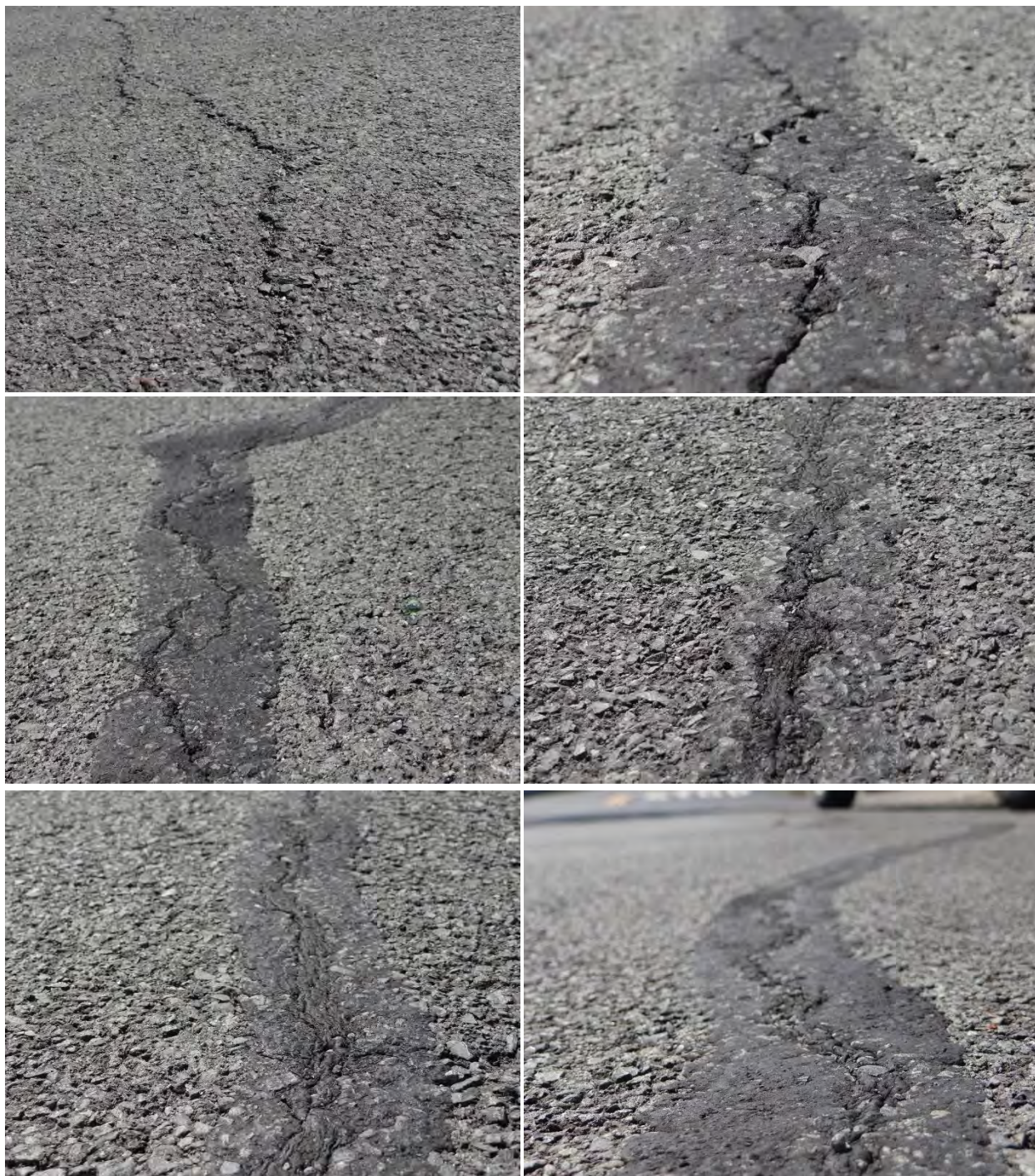
Figure C-33 Condition of the Kaweloka Place section on 01/26/2018.
