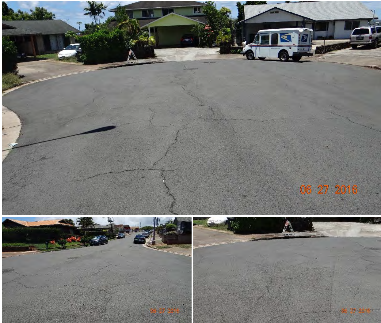
Figure C-24 Condition of the Palamoi Street section on 06/27/2016 (sixteen months into the study period) used as control for crack sealing.
