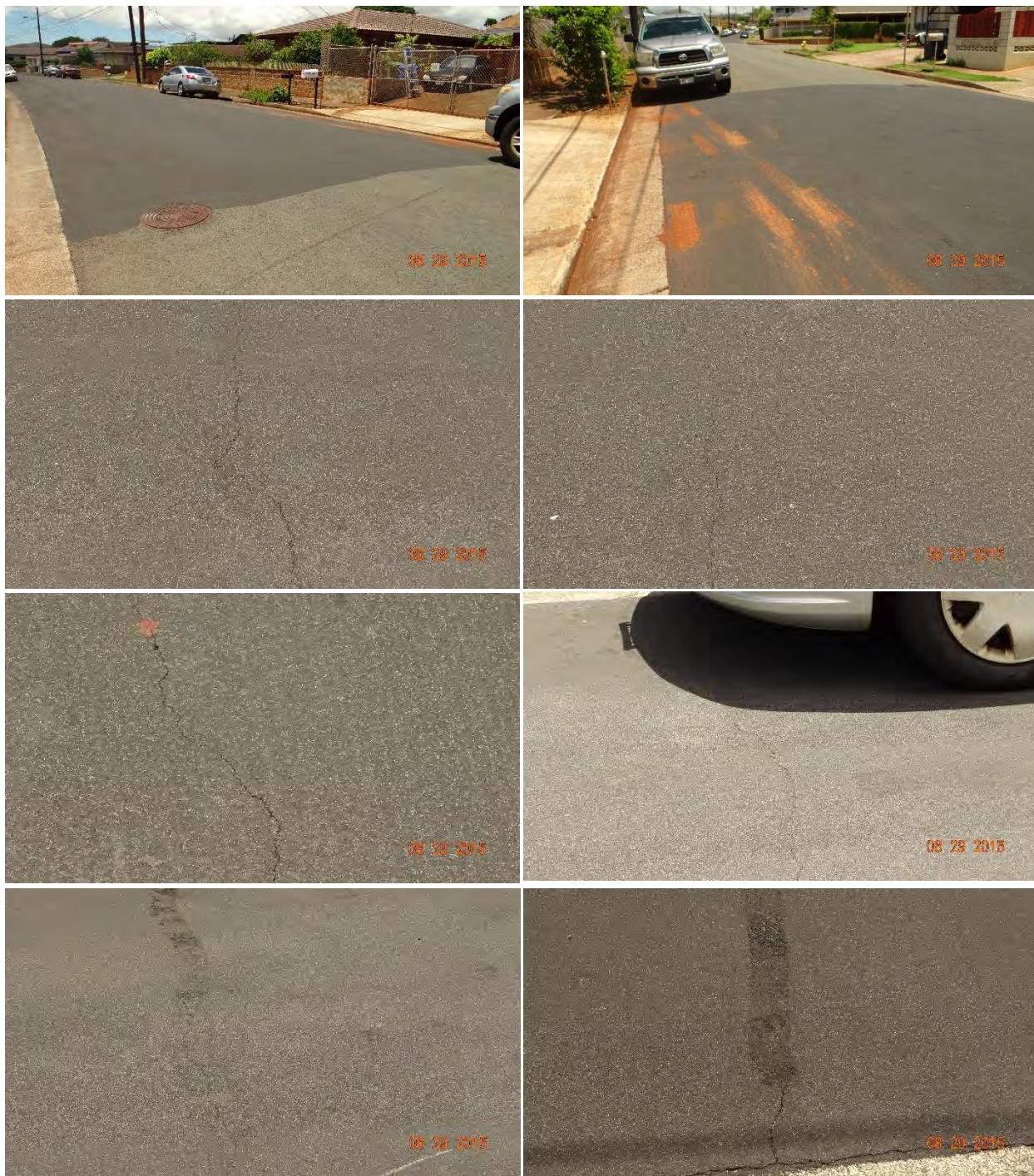
Figure C-61 Condition of Kaweloka Street section 2, treated with Liquid Road, on 8/29/2015.
