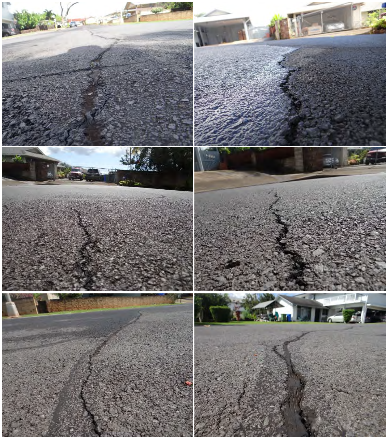
Figure C-44 Condition of the Paaaina Place section on 02/07/2018.
