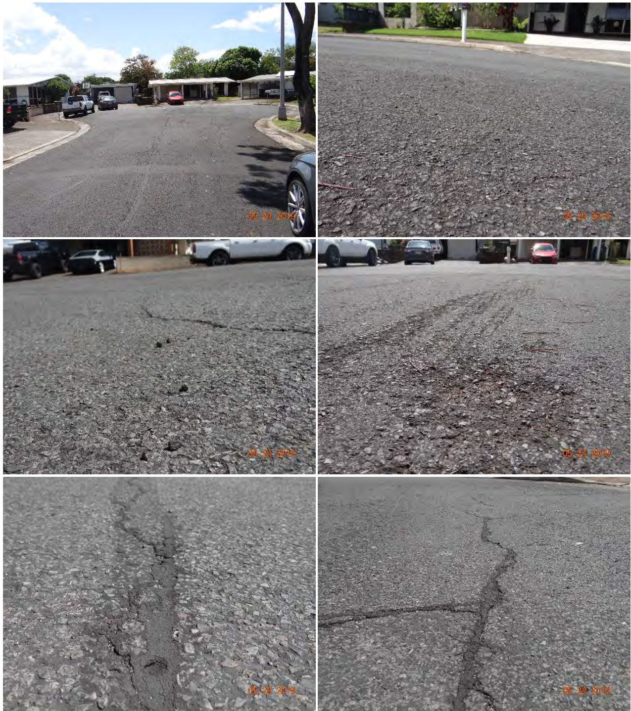
Figure C-138 Condition of the section on Hooheho Place, before treatment with CarbonSeal-HF by Carbonyte Systems Inc., on 5/24/2019.
