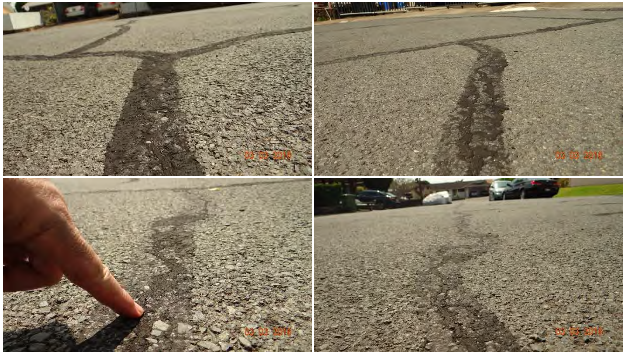
Figure C-27 Condition of the Kaweloka Place section on 03/03/2016.
