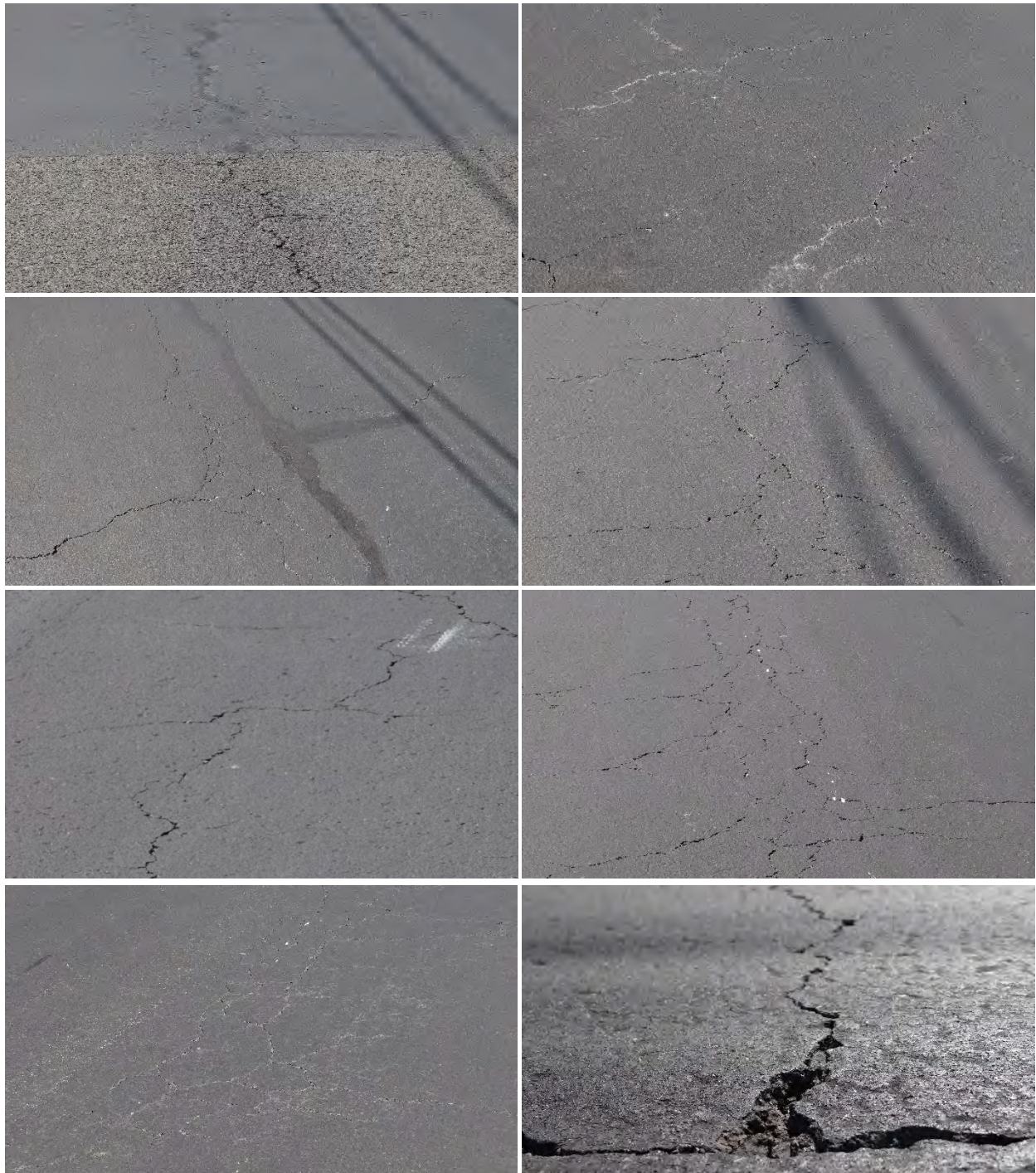
Figure C-81 Cracking on Kaweloka Street section 4, treated with OptiPave Plus™ RTU, on 1/26/2018.
