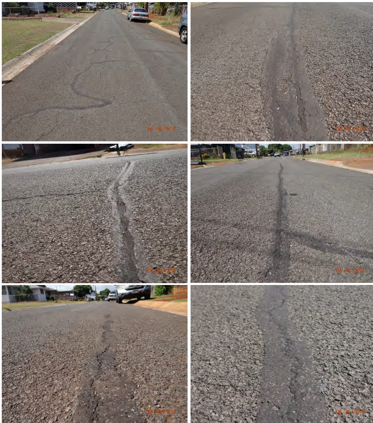
Figure C-10 Condition of crack sealing observed on Hoowali Street on 5/24/2019 (sealed with CrackMaster™ PL-HT).
