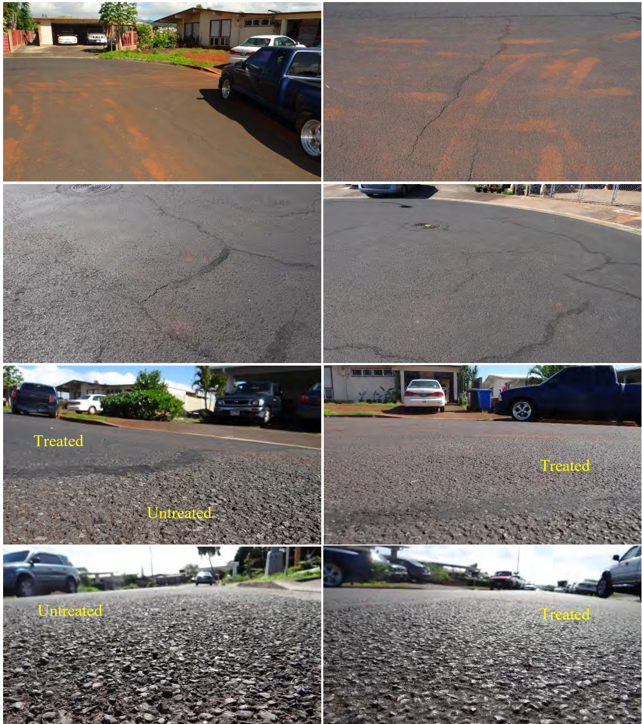
Figure C-122 Condition of the section on Hoolana Place, treated with OptiPave Plus™ Ready to Use by SealMasters®/Hawaii, on 12/14/2016.
