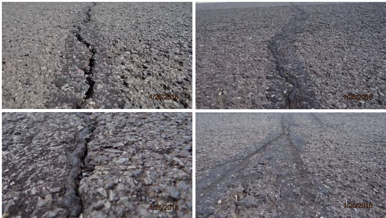
Figure C-19 Condition of crack sealing observed on Hookano Street on 01/26/2018 (sealed with Roadsaver 211).
