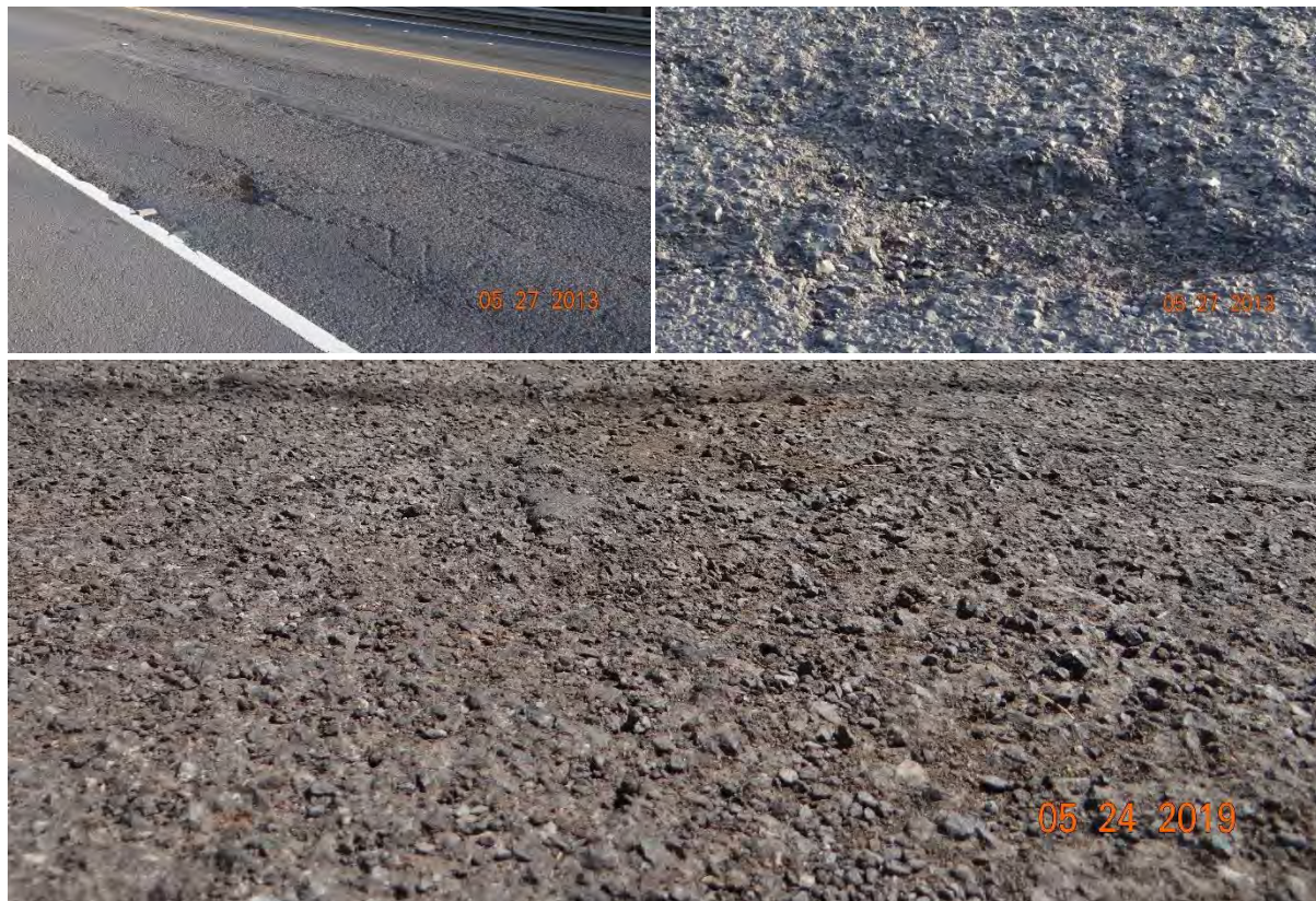
Figure 4-32. Illustrations of the disintegration of the pavement surface from severe raveling left untreated and the unsightly stop-gap repairs needed.
