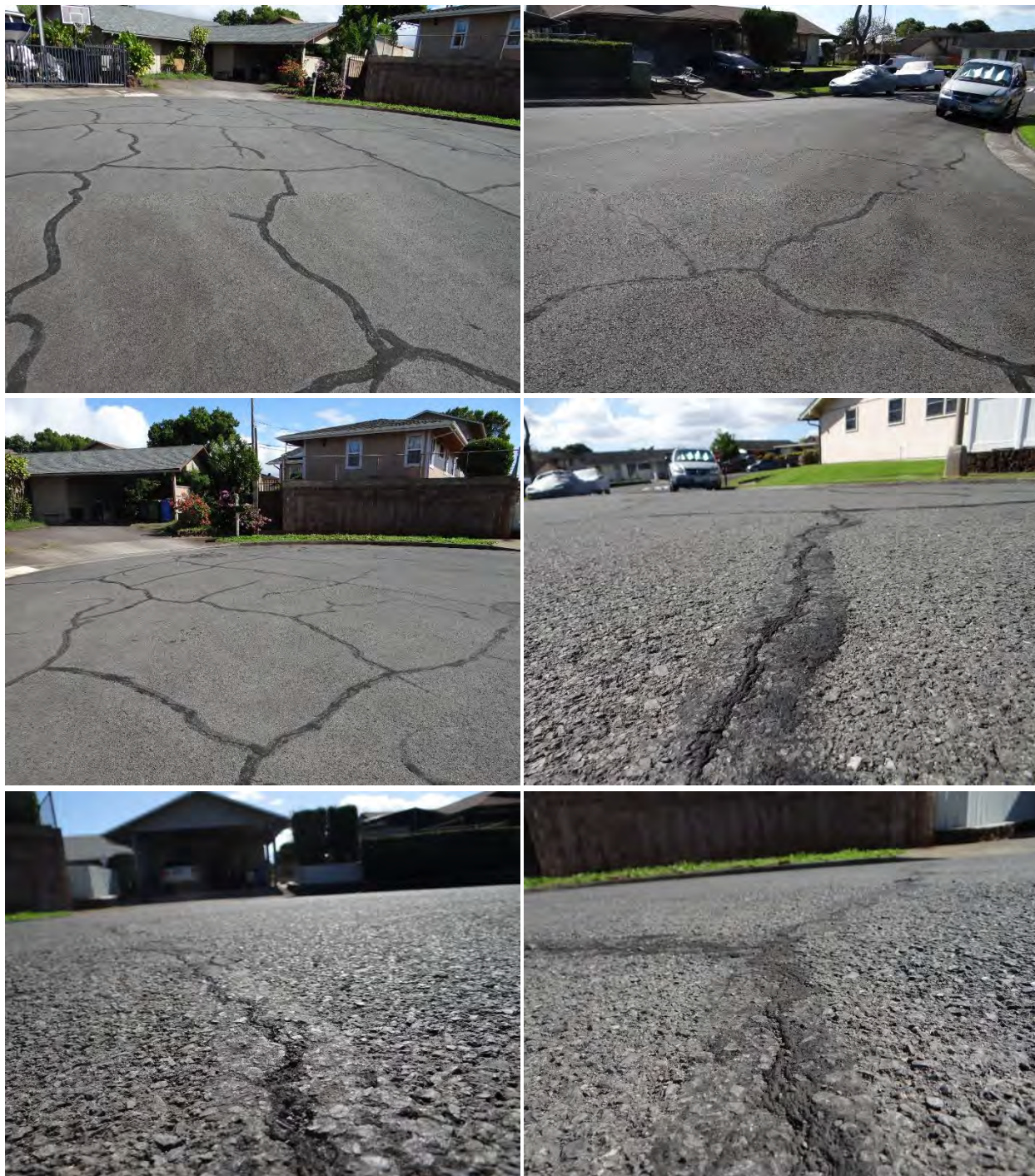
Figure C-30 Condition of the Kaweloka Place section on 12/14/2016.
