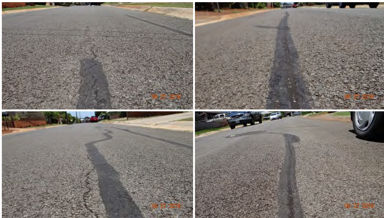
Figure C-7 Condition of crack sealing observed on Hoowali Street on 06/27/2016 (sealed with CrackMaster™ PL-HT).
