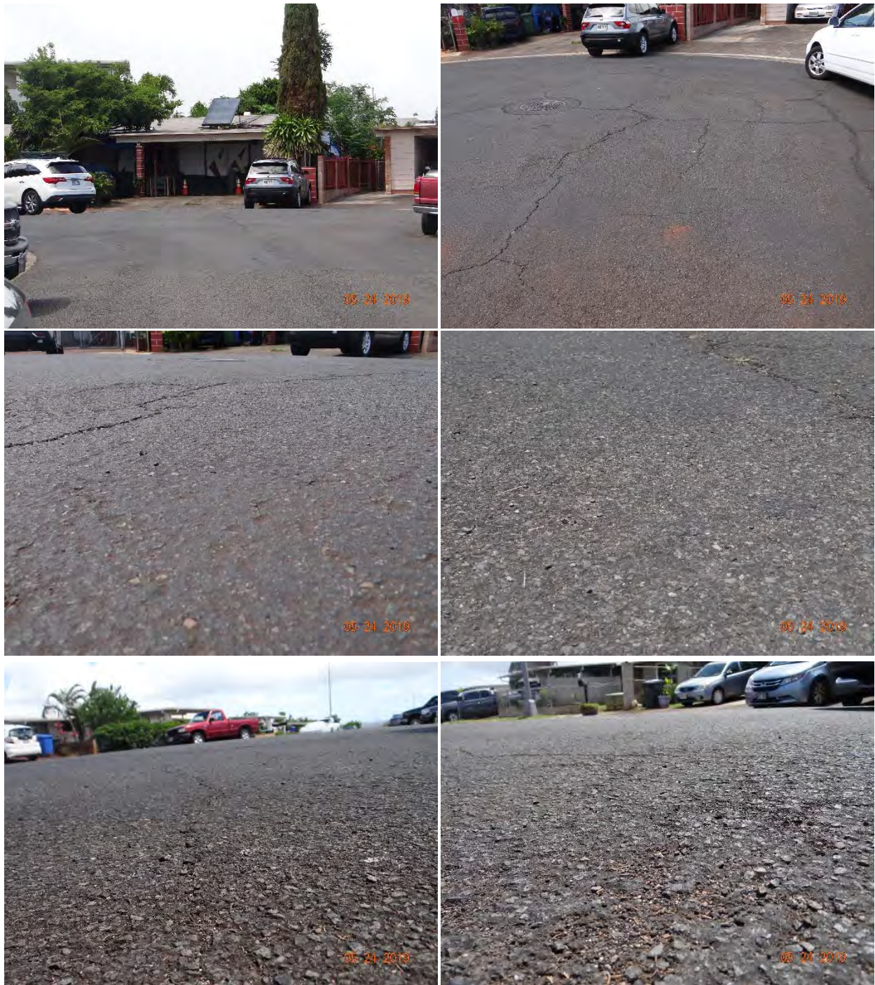
Figure C-124 Condition of the section on Hoolana Place, treated with OptiPave Plus™ Ready to Use by SealMasters®/Hawaii, on 5/24/2019.
