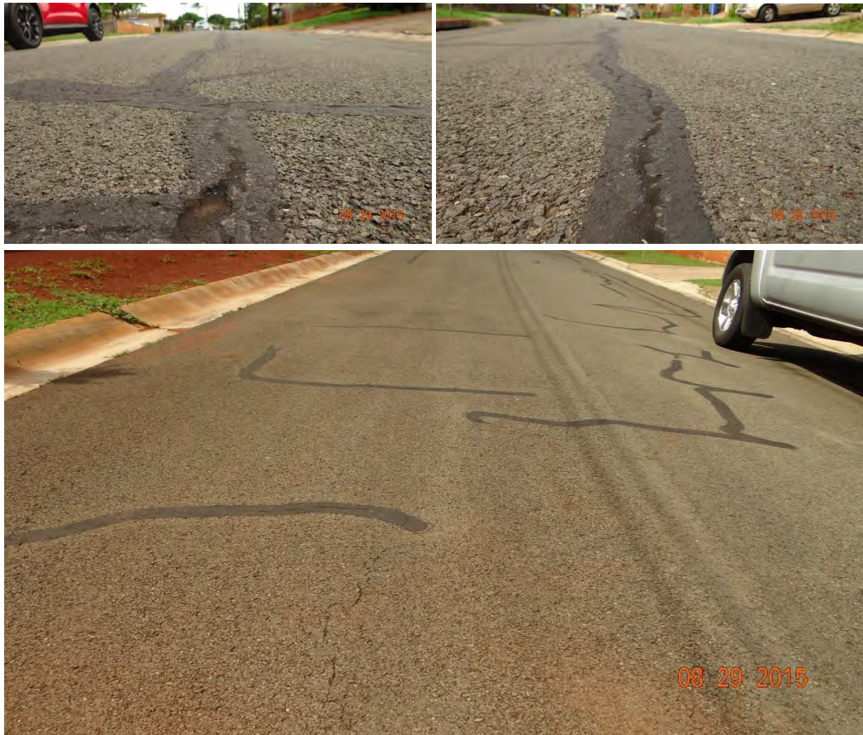
Figure C-5 Cracking patterns observed on Hoowali Street on 08/29/2015 (sealed with CrackMaster™ PL-HT).
