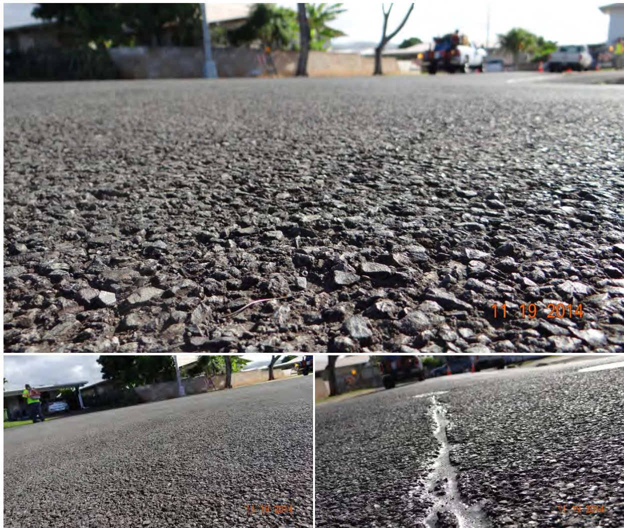
Figure C-132 Surface condition on Hooheno Place, before treatment with CarbonSeal-HF by Carbonyte Systems Inc., on 11/19/2014.
