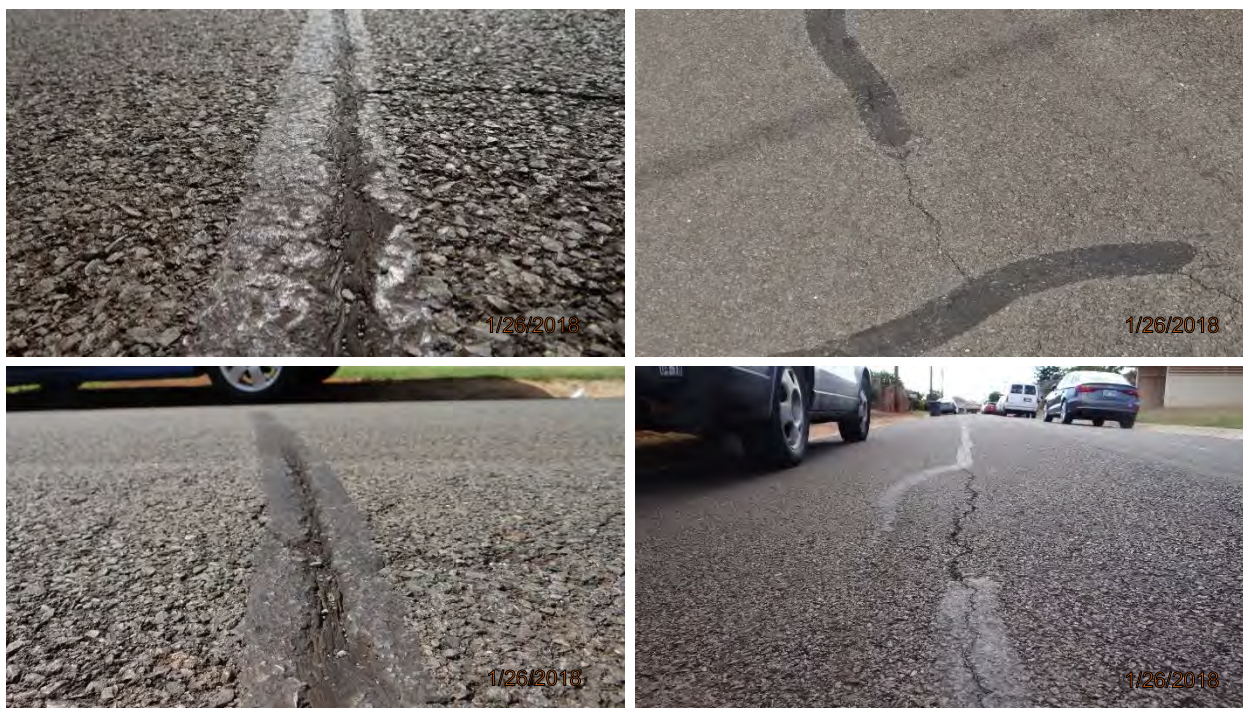
Figure C-8 Condition of crack sealing observed on Hoowali Street on 01/26/2018 (sealed with CrackMaster™ PL-HT).
