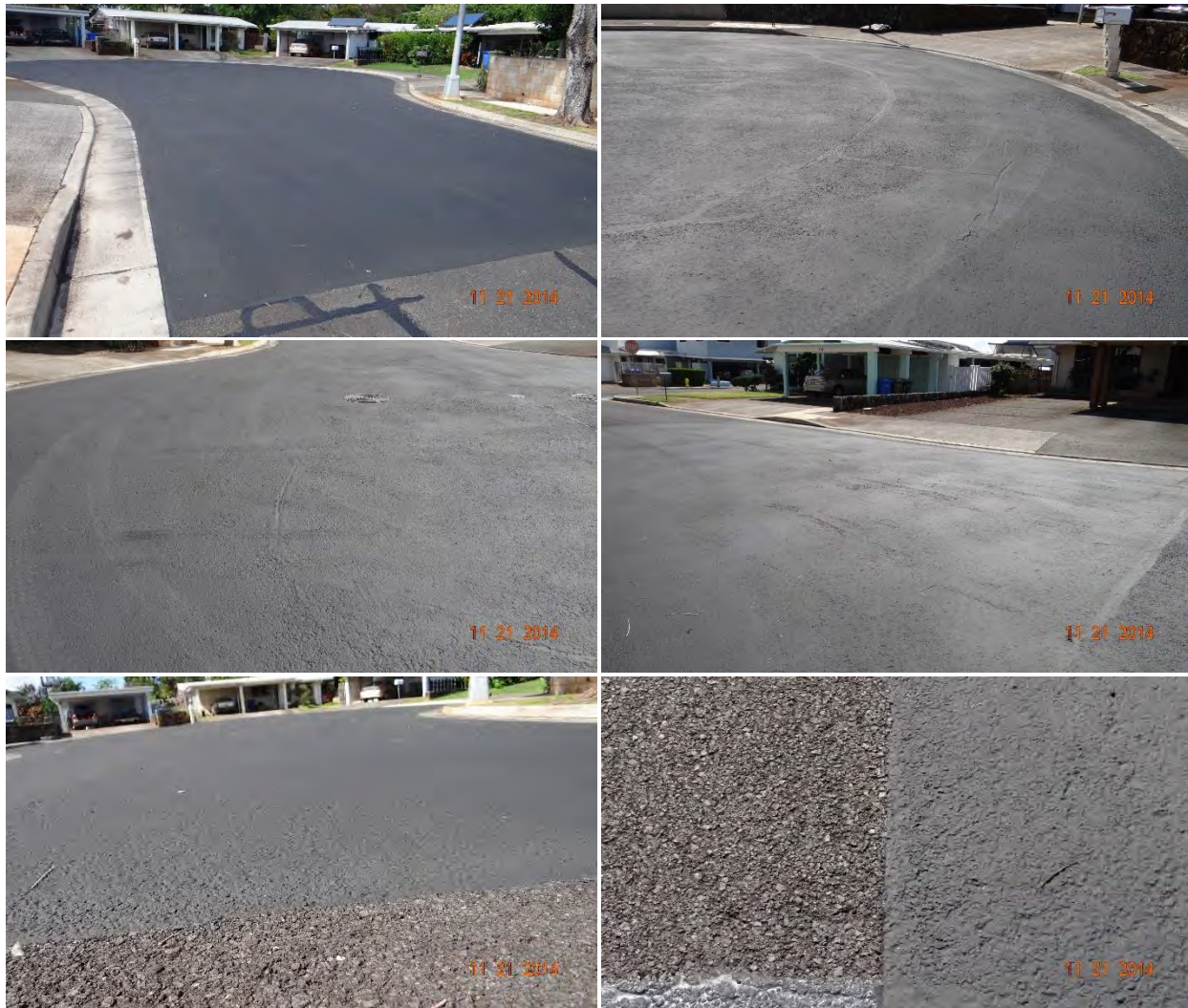
Figure C-133 Condition of the section on Hooheno Place, before treatment with CarbonSeal-HF by Carbonyte Systems Inc., on 11/21/2014.
