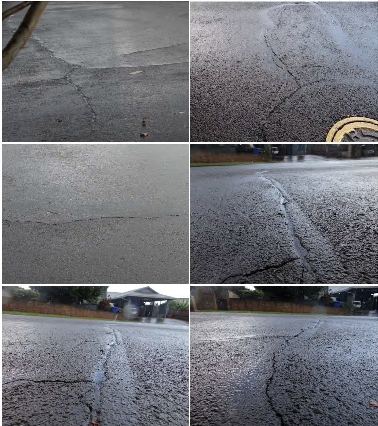
Figure C-47 Condition of the Paaaina Place section on 02/07/2018.
