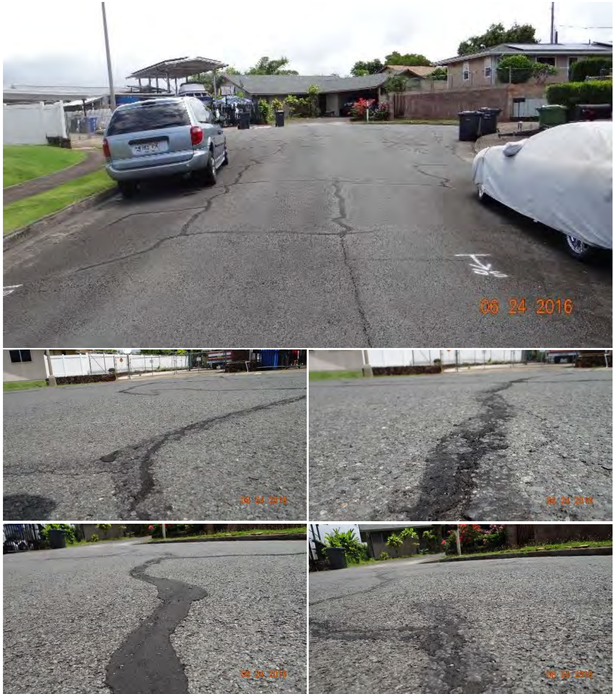
Figure C-28 Condition of the Kaweloka Place section on 06/24/2016.
