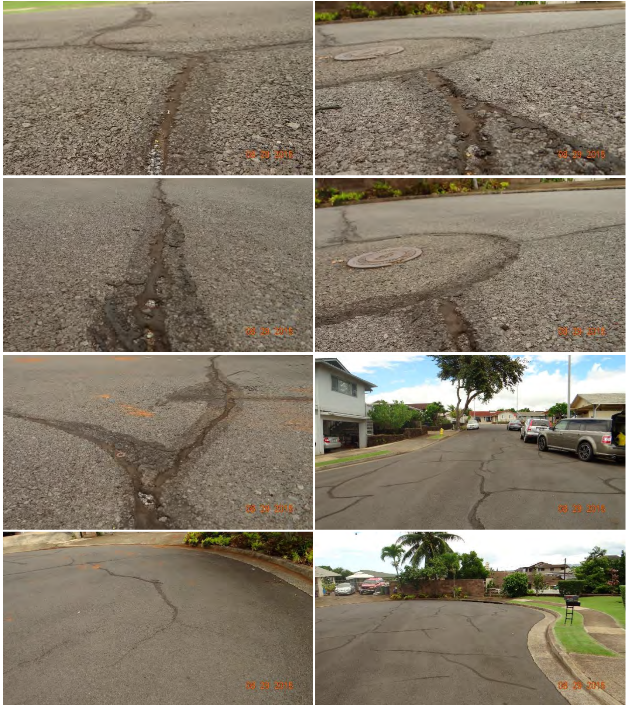
Figure C-38 Condition of the Paaaina Place section on 08/29/2015.
