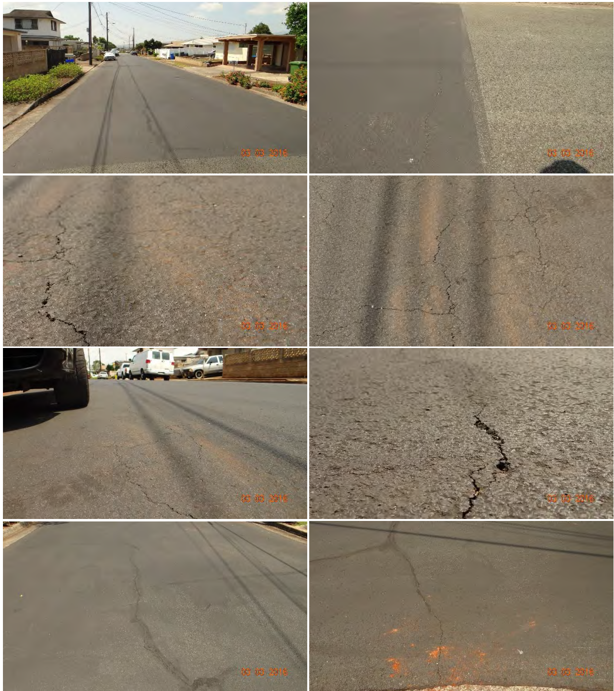
Figure C-78 Condition of Kaweloka Street section 4, treated with OptiPave Plus™ RTU, on 3/3/2016.
