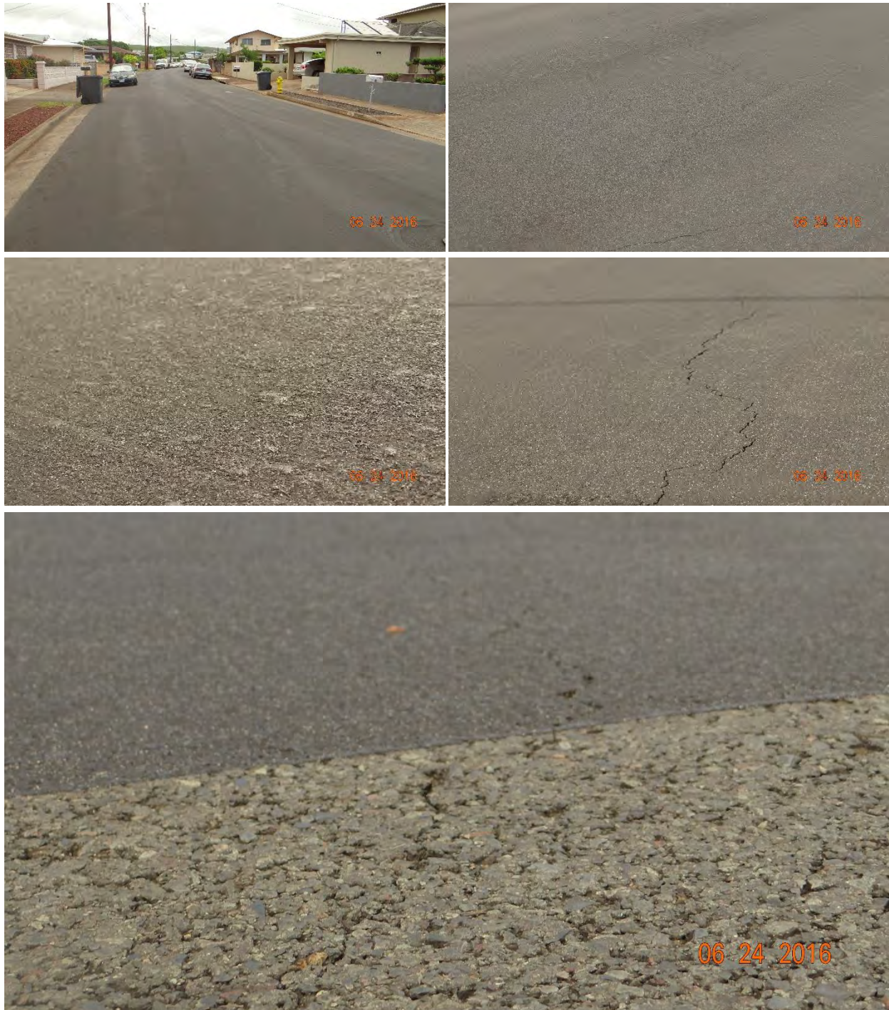
Figure C-64 Condition of Kaweloka Street section 2, treated with Liquid Road, on 6/24/2016.
