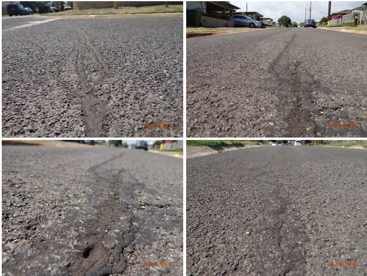
Figure C-22 Condition of crack sealing observed on Hookano Street on 5/24/2019 (sealed with Roadsaver 211).
