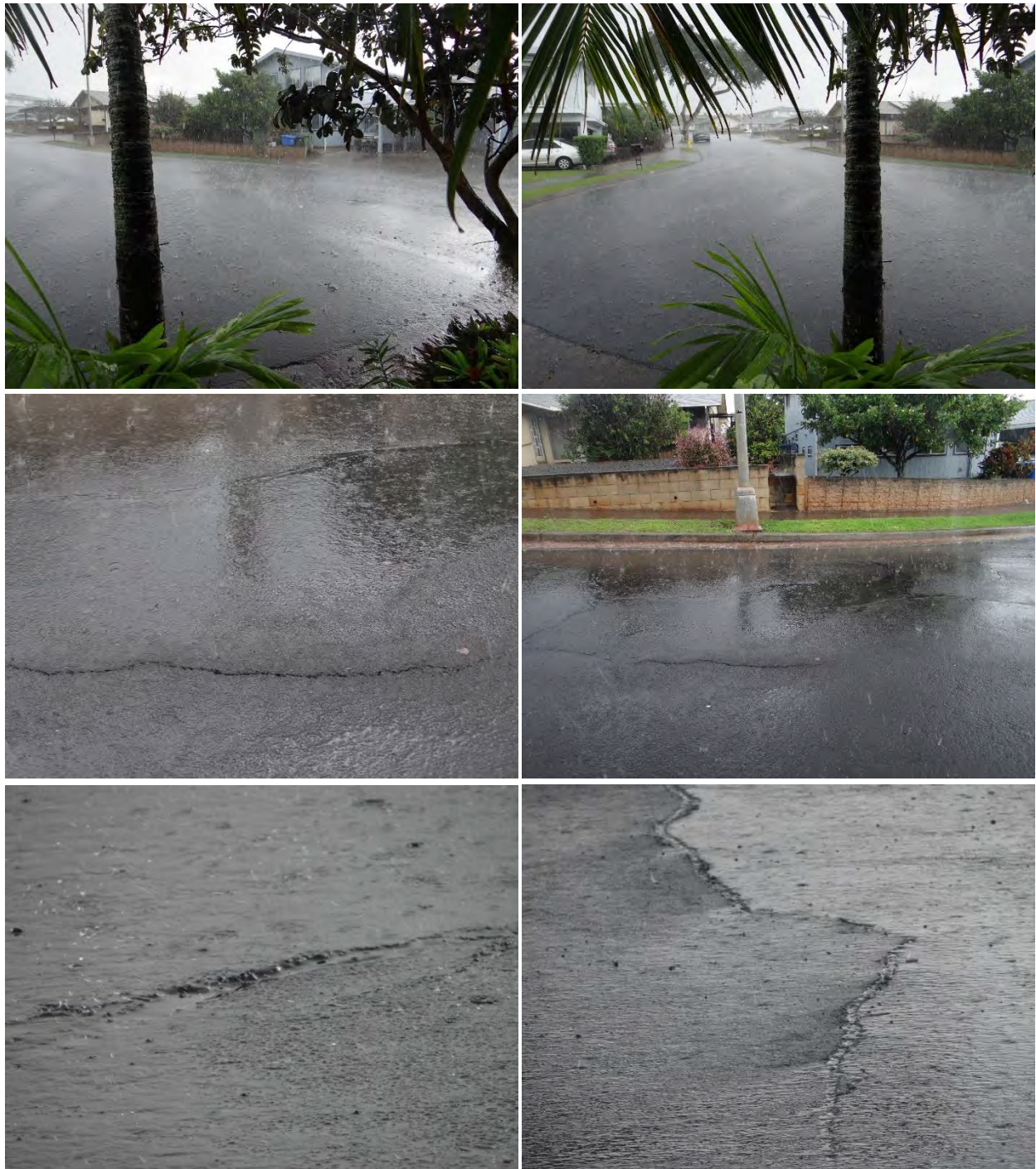
Figure C-46 Condition of the Paaaina Place section on 02/07/2018.
