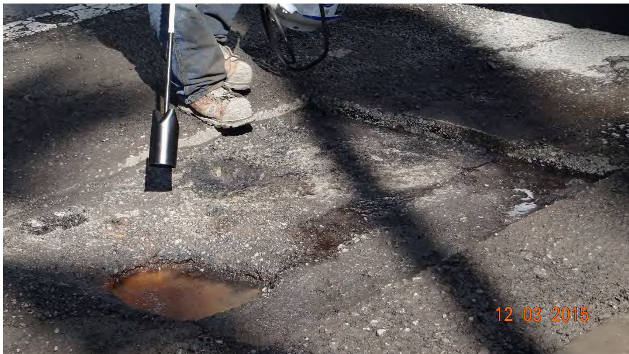
Figure 4-16 Example of water raising from underlying layers through a pothole in a road with high longitudinal slope.
