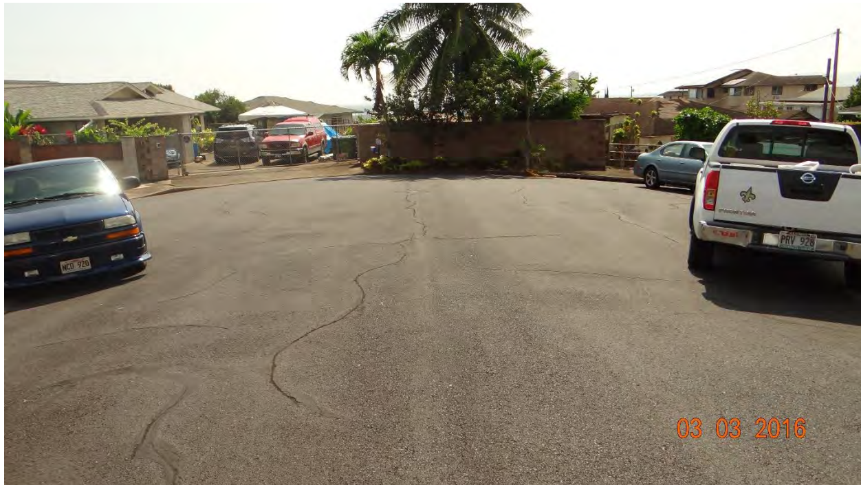
Figure C-40 Condition of the Paaaina Place section on 03/03/2016.
