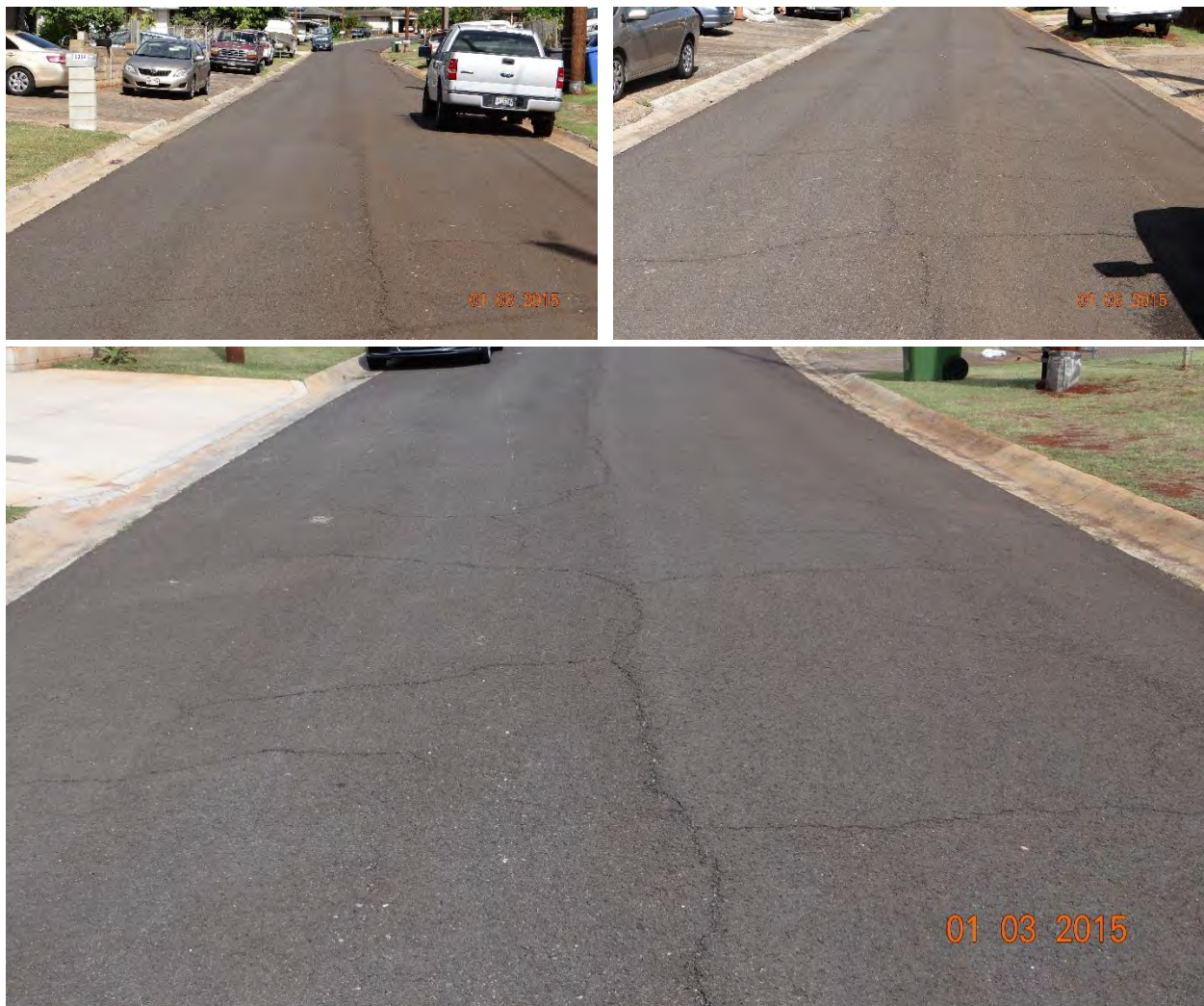
Figure C-1 Cracking patterns observed on the Control Section on Hoolauna Street on 01/03/2015.
