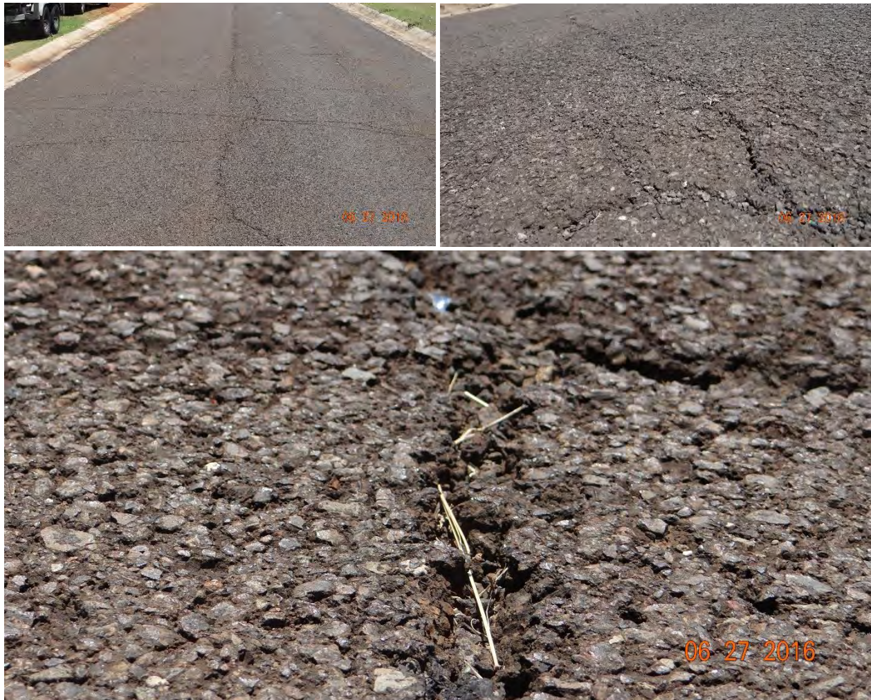
Figure C-3 Cracking patterns observed on the Control Section on Hoolauna Street on 06/27/2016.
