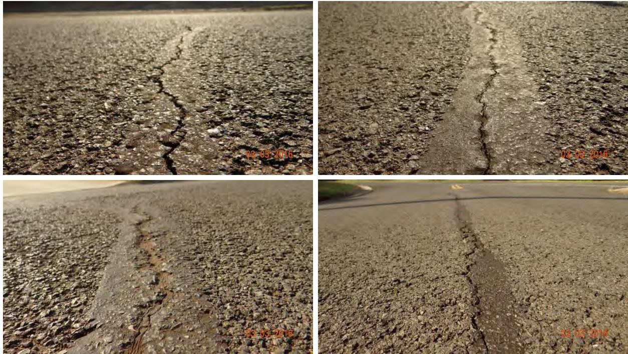
Figure C-16 More on the condition of crack sealing observed on Hookano Street on 03/03/2016 (sealed with Roadsaver 211).
