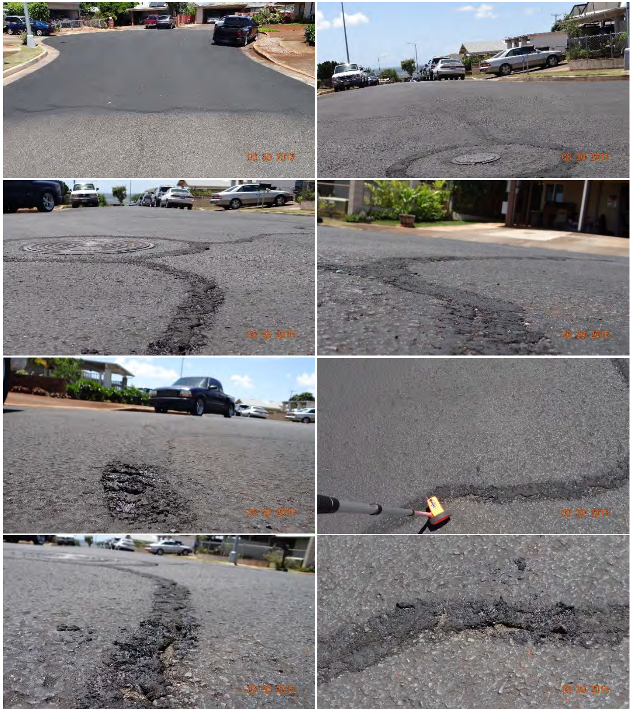
Figure C-118 Condition of the section on Hoolana Place, treated with OptiPave Plus™ Ready to Use by SealMasters®/Hawaii, on 3/30/2015.
