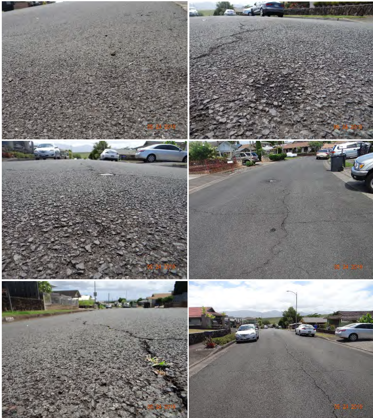
Figure C-86 Condition of control sections 6, 7, 8 for straight sections without bus traffic on Kaweloka Street, on 5/24/2019.
