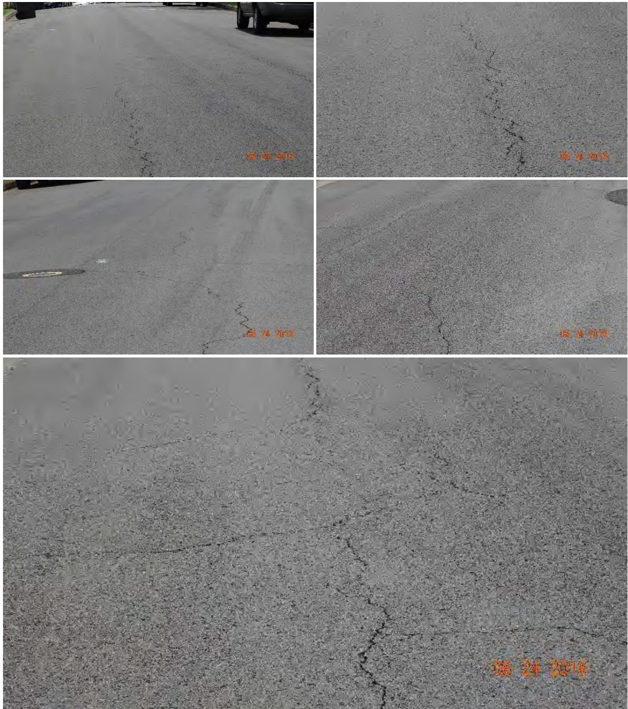
Figure C-84 Condition of control sections 6, 7, 8 for straight sections without bus traffic on Kaweloka Street, on 6/24/2016.
