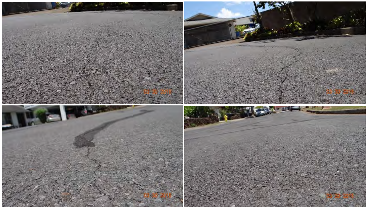
Figure C-37 Condition of the Paaaina Place section on 03/30/2015.
