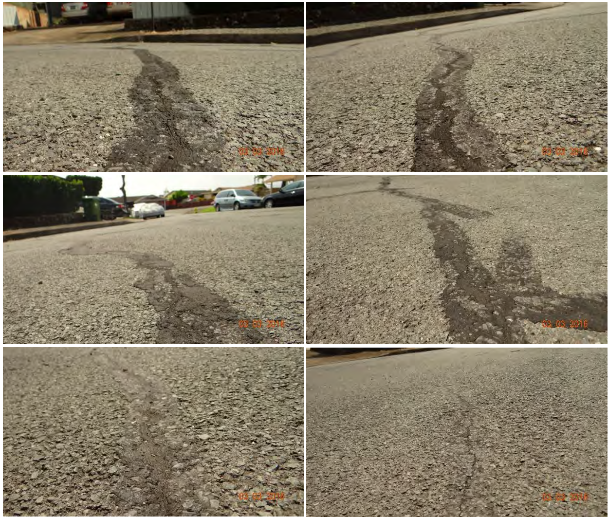
Figure C-26 Condition of the Kaweloka Place section on 03/03/2016.
