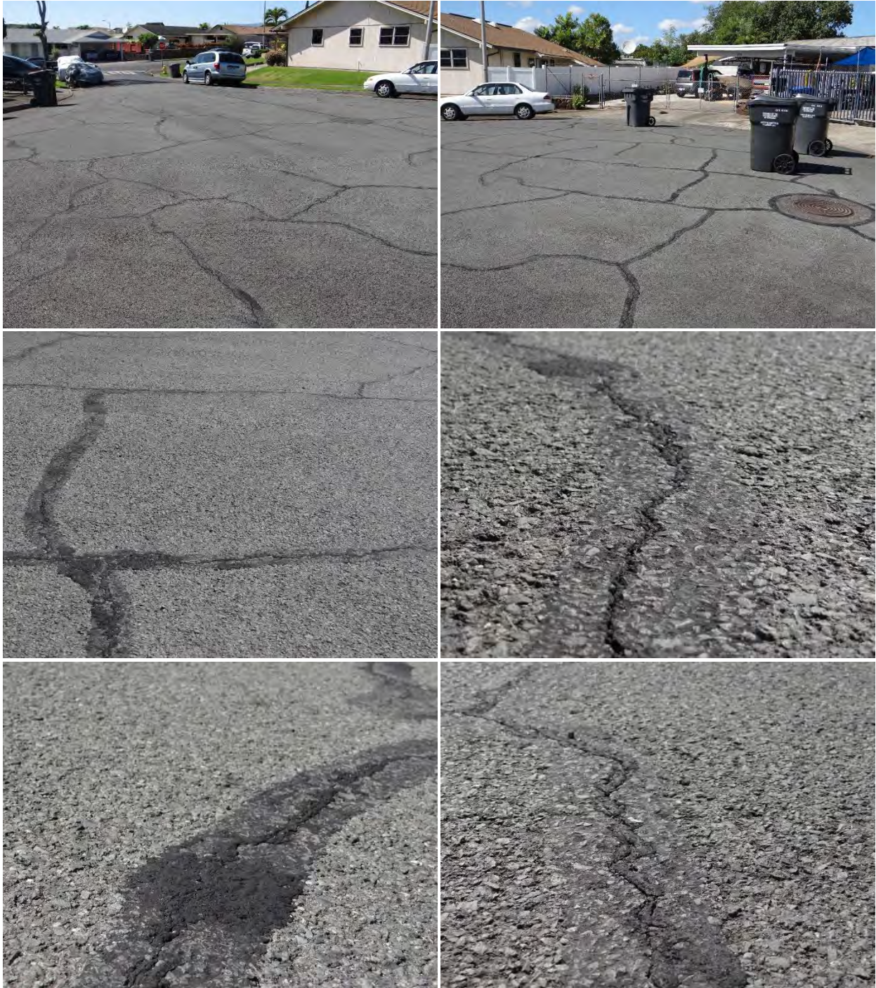
Figure C-32 Condition of the Kaweloka Place section on 01/26/2018.
